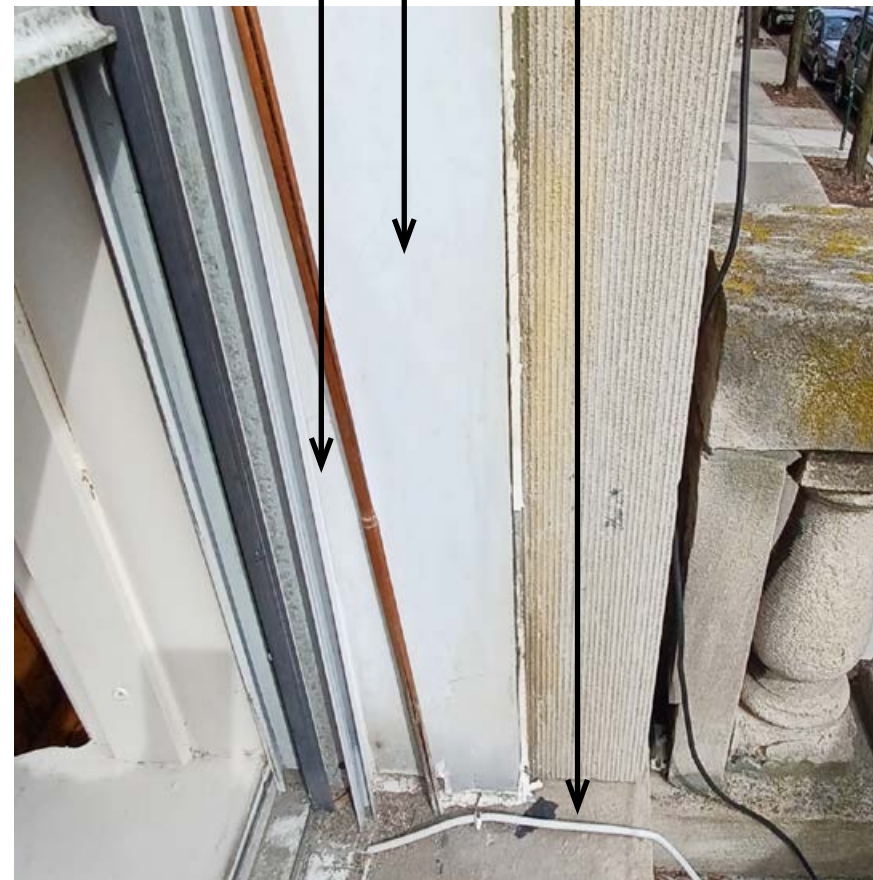
Existing Window C (typ.) - window unit, aluminum jambs to be removed. Original limestone sill to remain.
