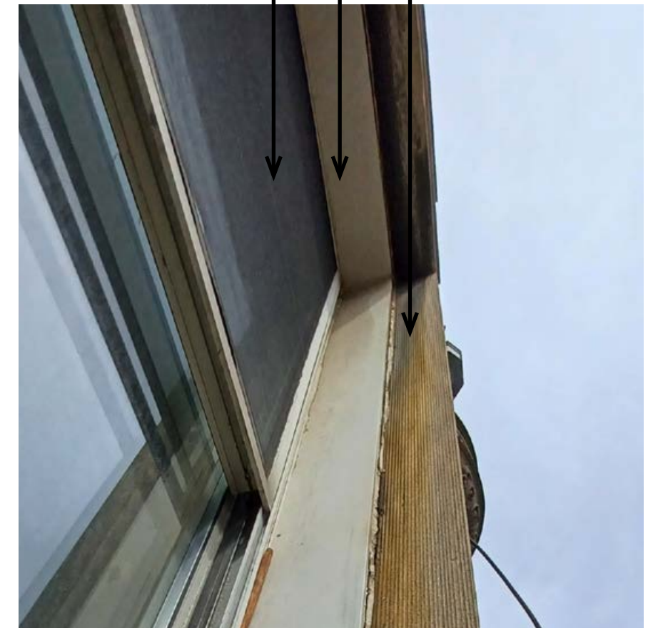
Existing Window C (typ.) - window unit, aluminum clad jambs & head to be removed. Original limestone surrounds to remain.
