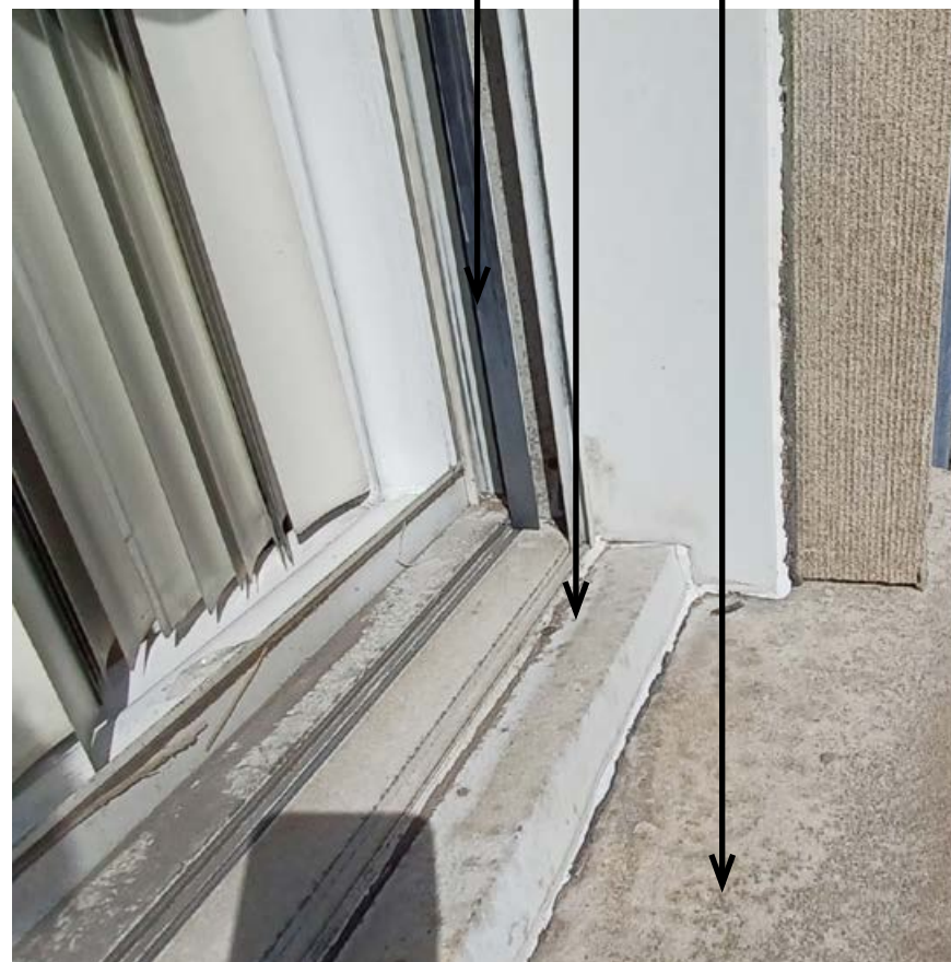
Existing Window D (typ.) - window unit, aluminum clad sill & jambs to be removed. Original limestone sill to remain.
