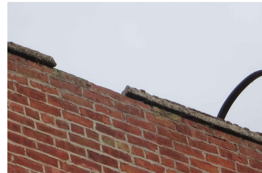
11 MISSING COPING STONE AT WEST FACADE
