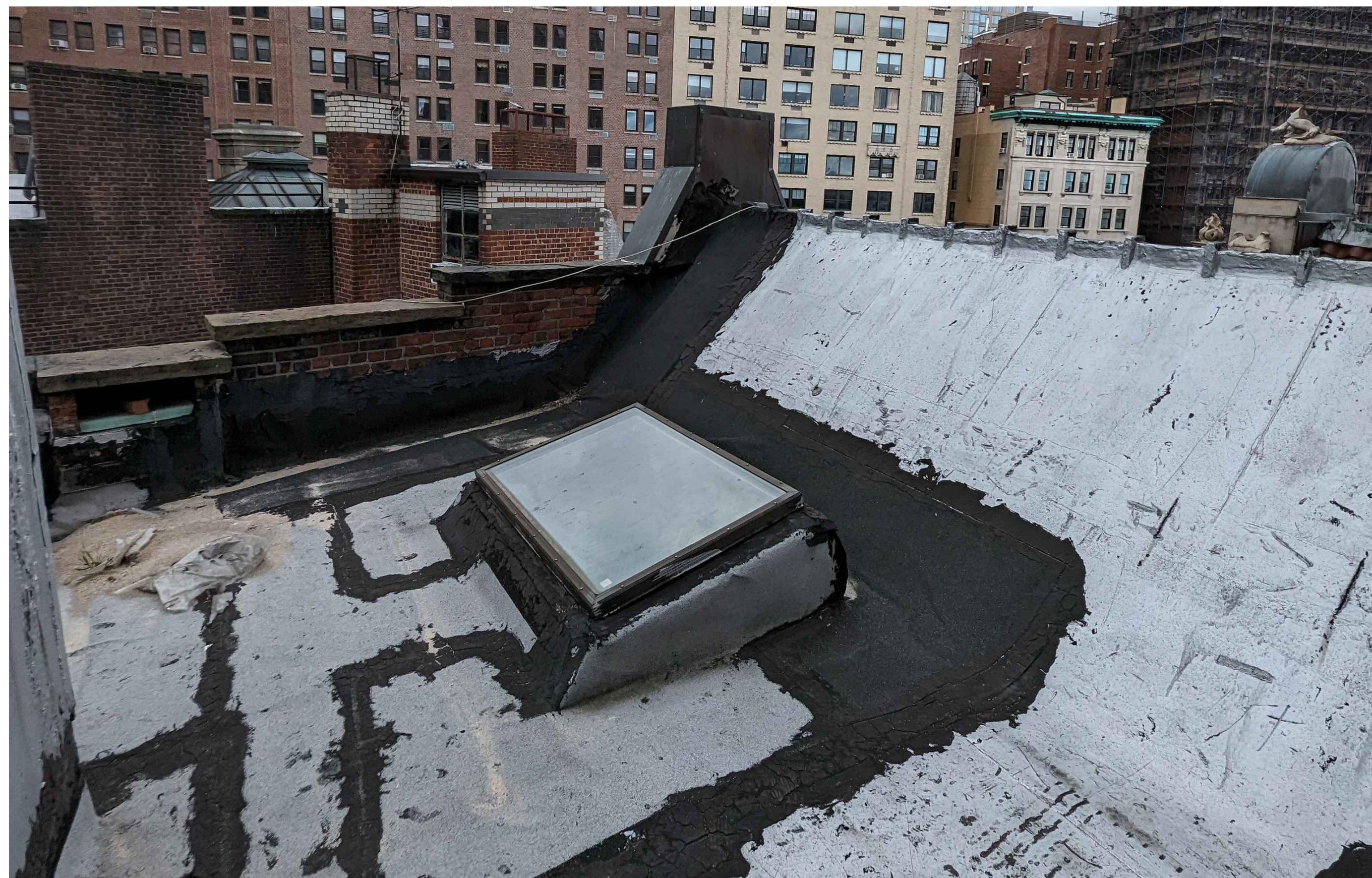
3 PHOTO OF EXISTING ROOF CONDITION SCALE: N.T.S.
