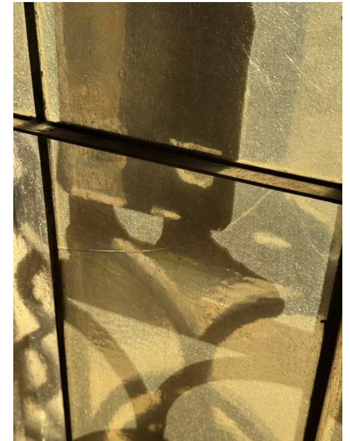
Broken Window Pane- Mezzanine
