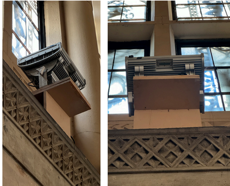
Non-original lighting to be removed
