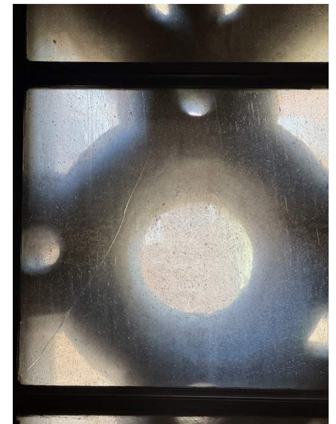
Broken Window Pane- Ground Floor
