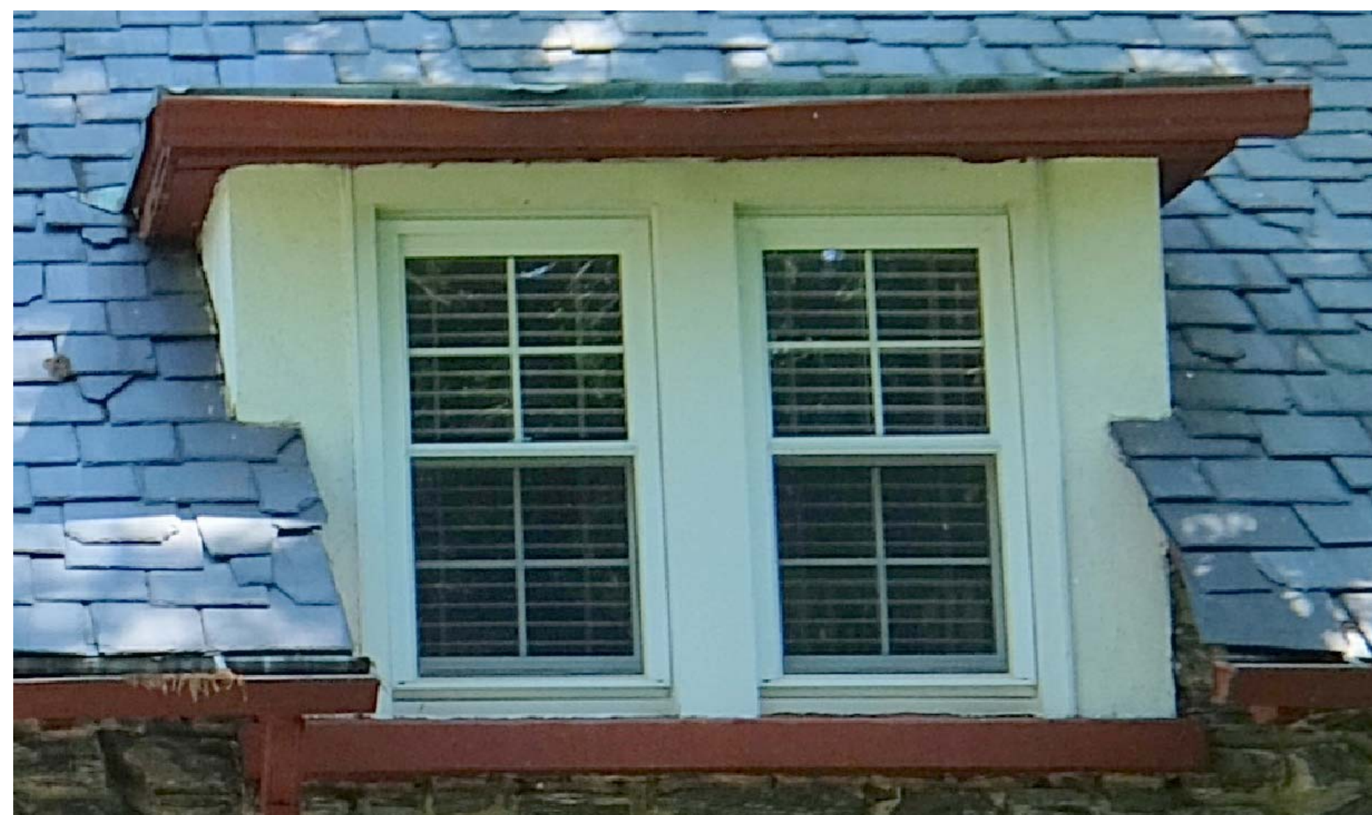
EXISTING 2ND FLOOR DORMER WINDOW VINYL WINDOWS TO BE REPLACED
