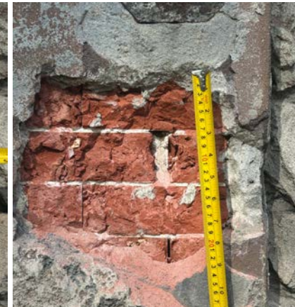
Brick probes showed that the removal of the cemented stone facade will damage the existing bricks face.
