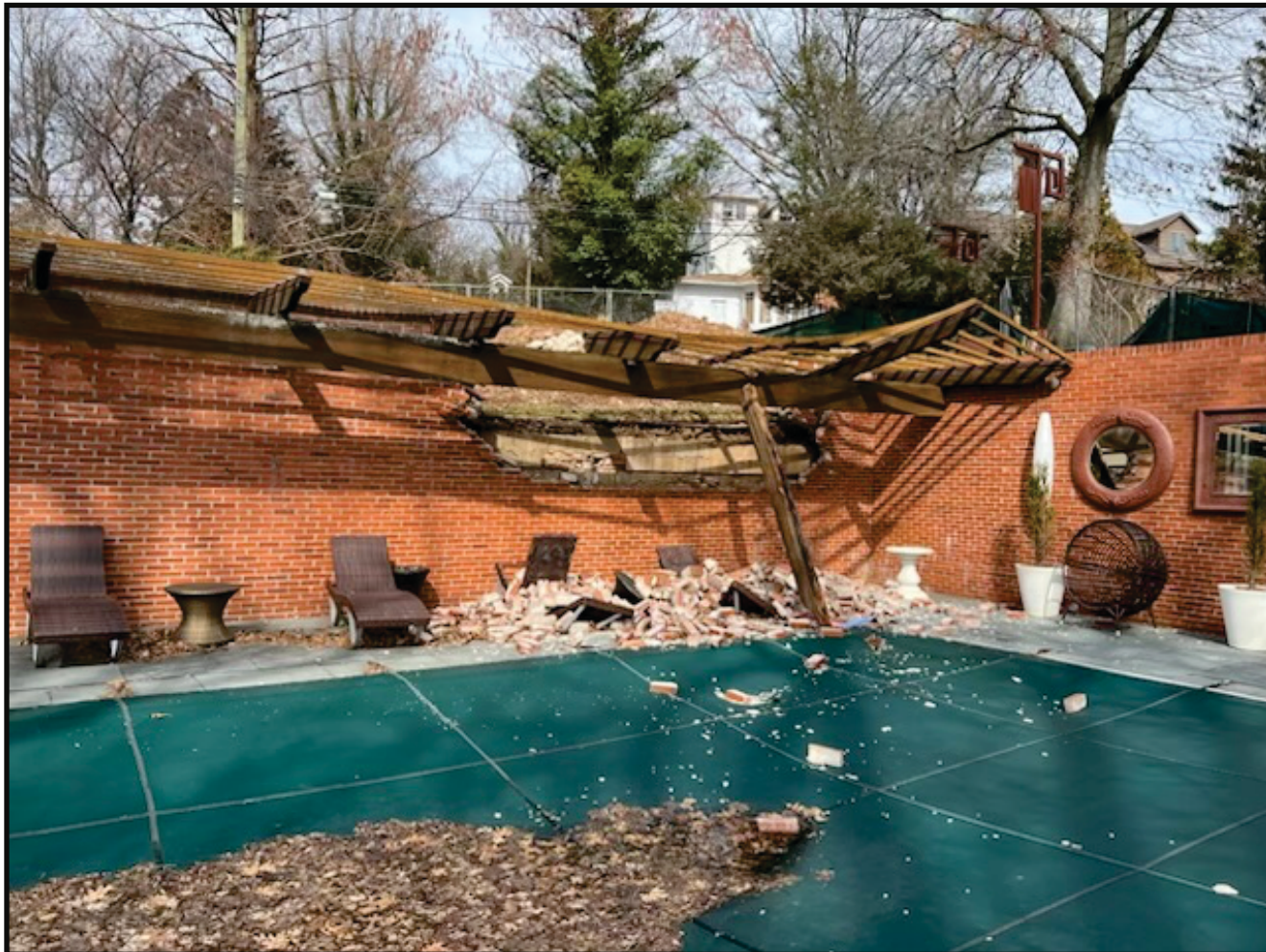
Photograph showing compromised retaining wall
