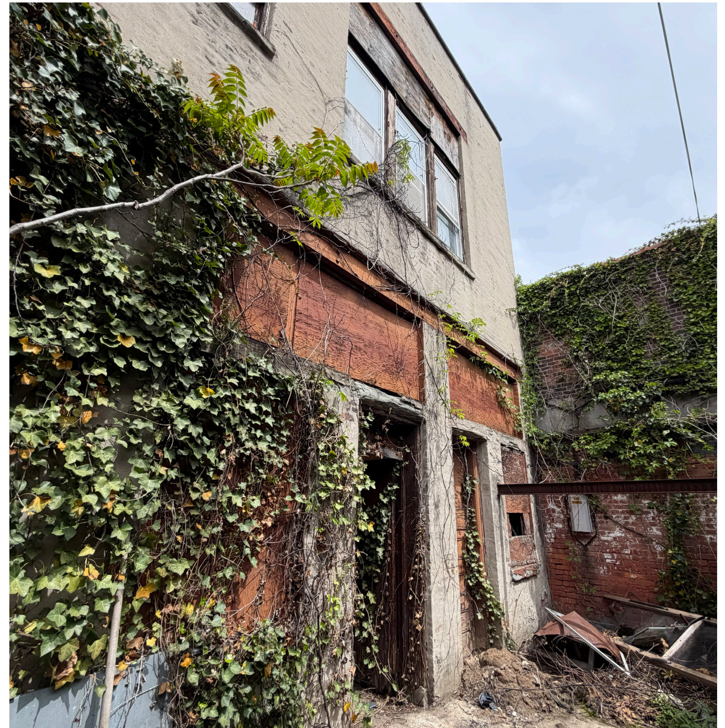
Rear of 144 Greenpoint (firestation). Facade will be demolished at rear of site. Rear facade contains no existing historical detailing or significance.
