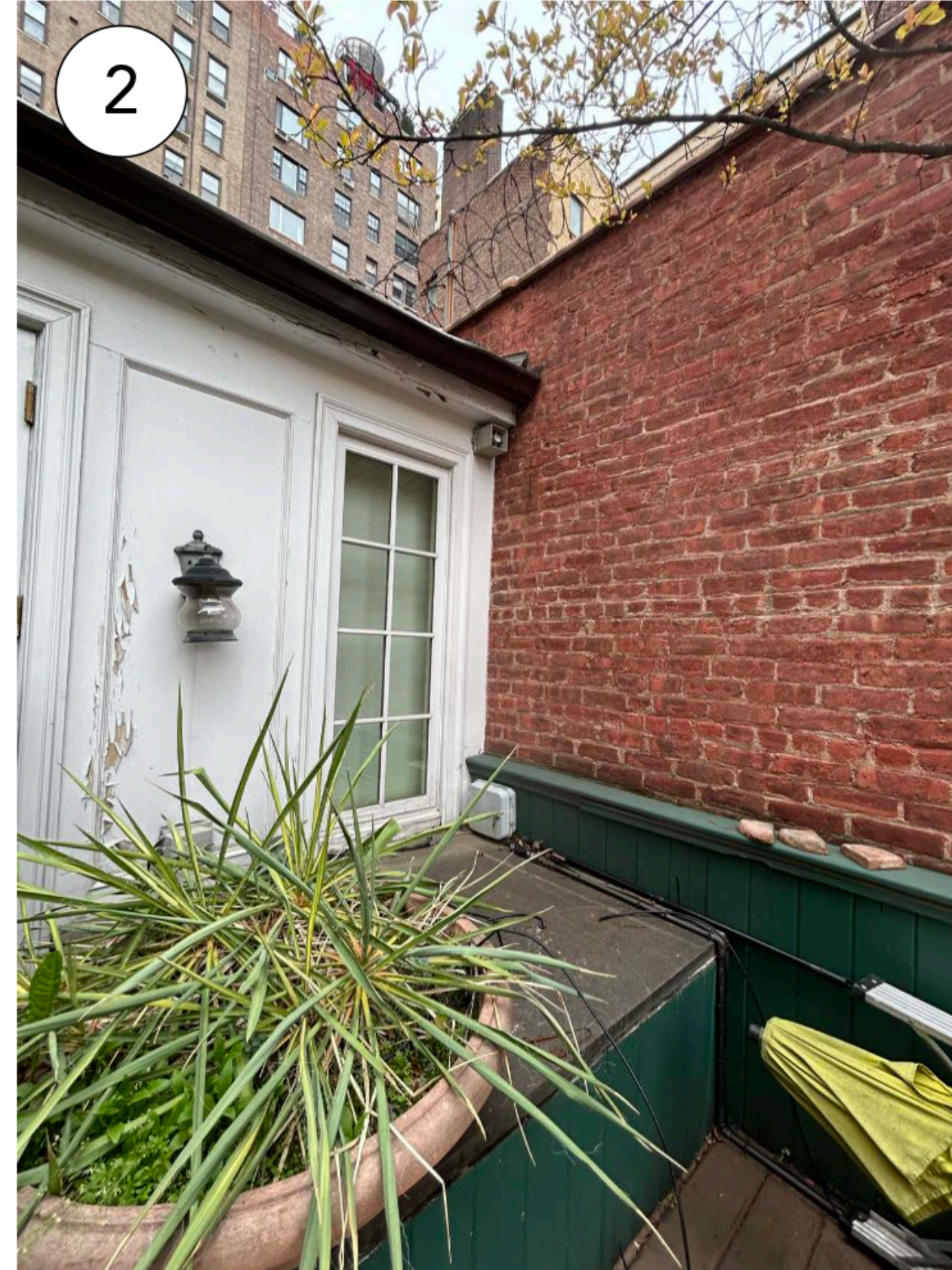
2 Flaking paint and a deteriorated gutter at the penthouse facade
