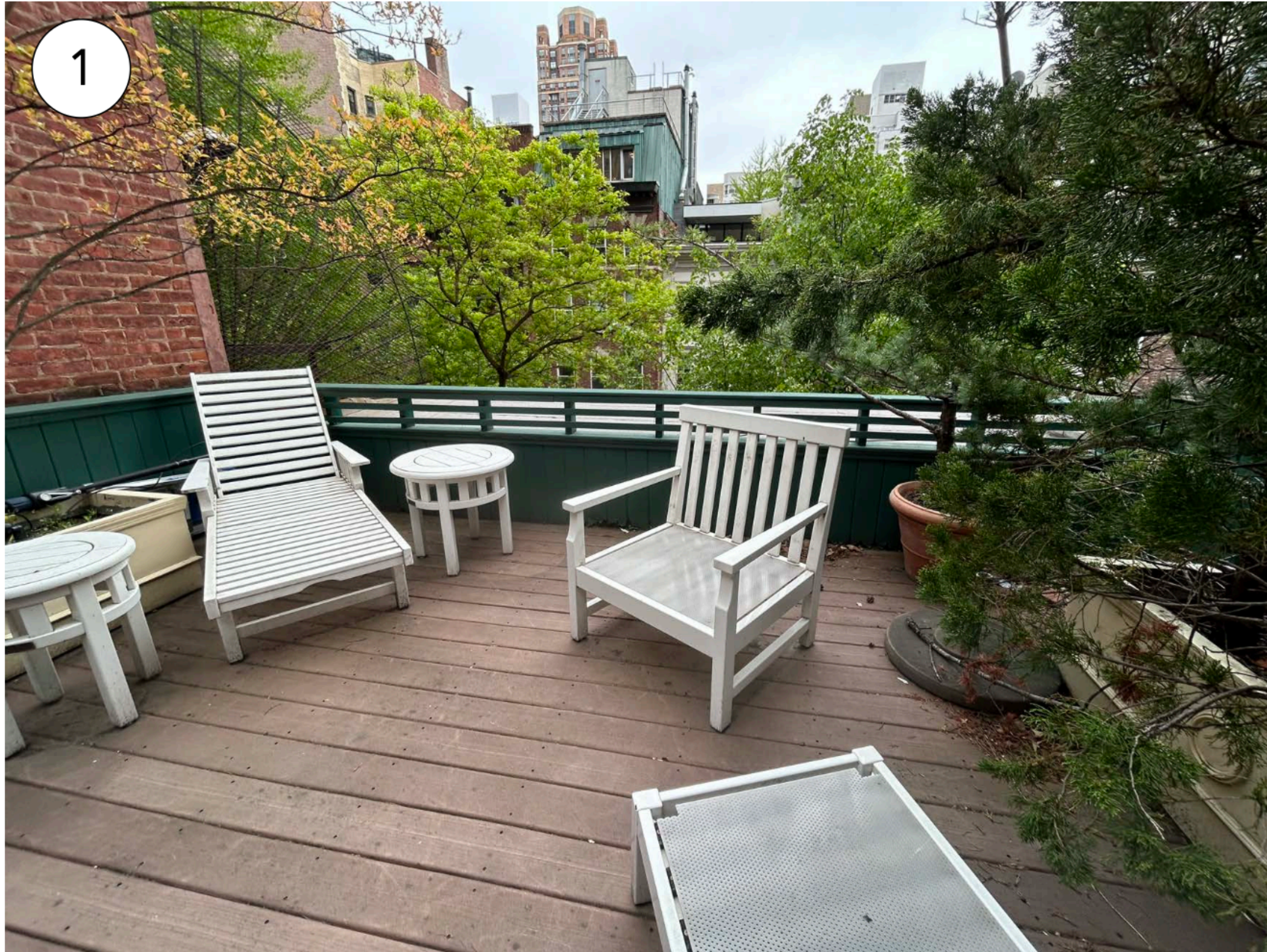
1 View to the southeast at the fourth floor roof terrace. Areas of water infiltration observed around perimeter and at interior of house
