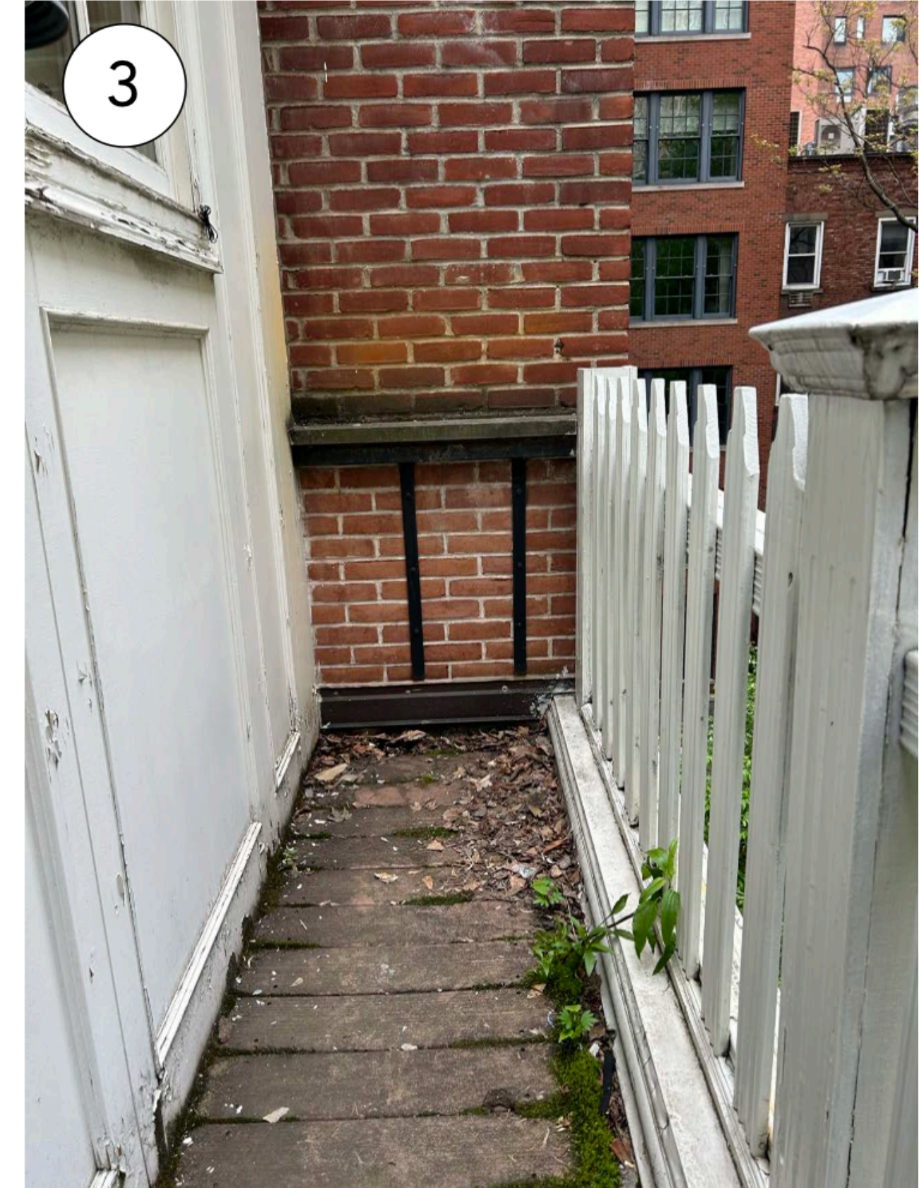
3 North side of penthouse addition with biological growth and damage to the wood decking
