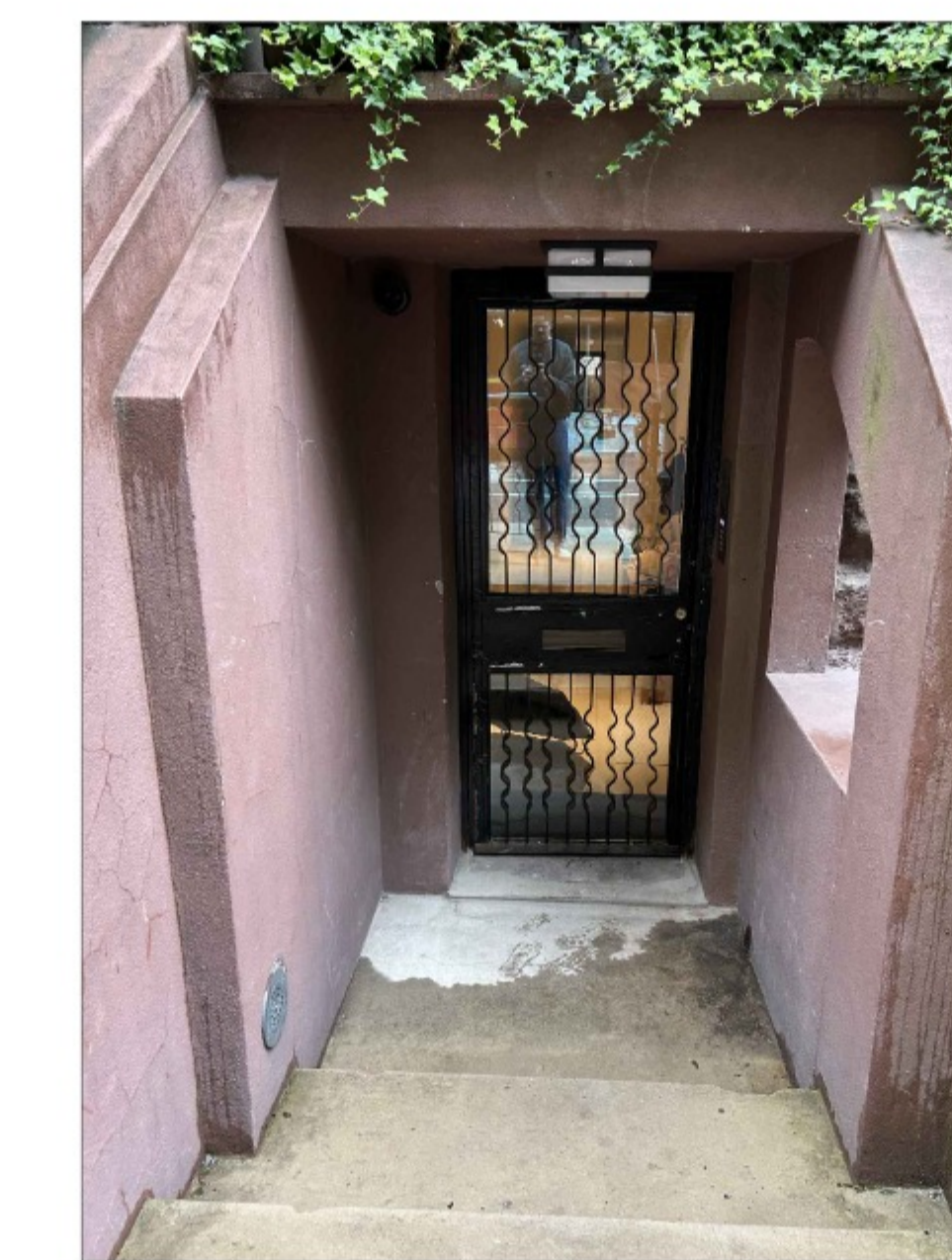
CURRENT WATER ISSUES @ AREAWAY MKCA RECORDS 10
