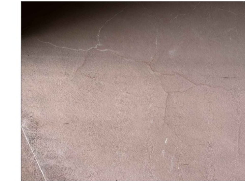
DAMAGED PARTS THROUGHOUT THE FACADE MKCA RECORDS 30
