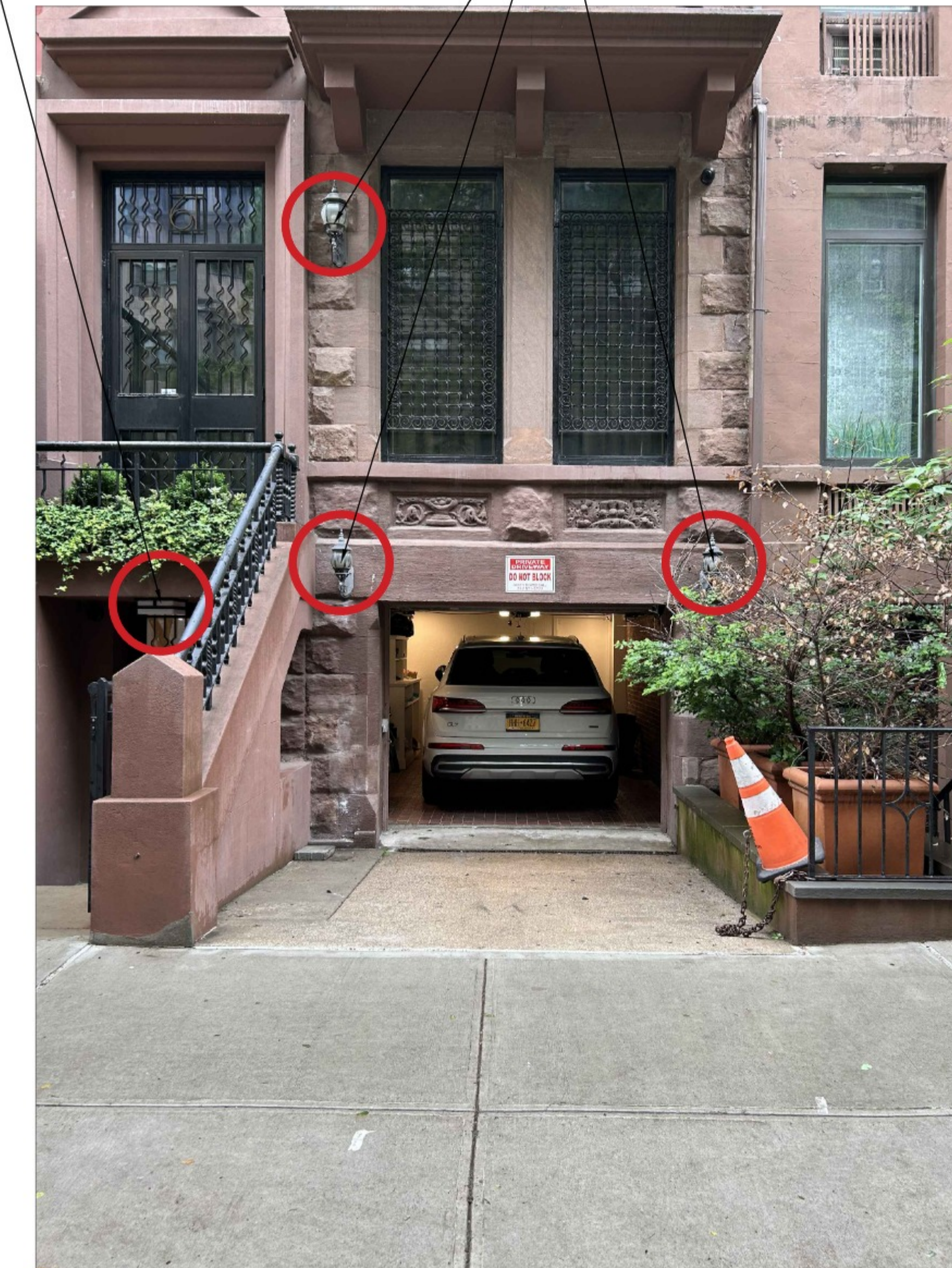
EXISTING LIGHT FIXTURES MKCA RECORDS 10
