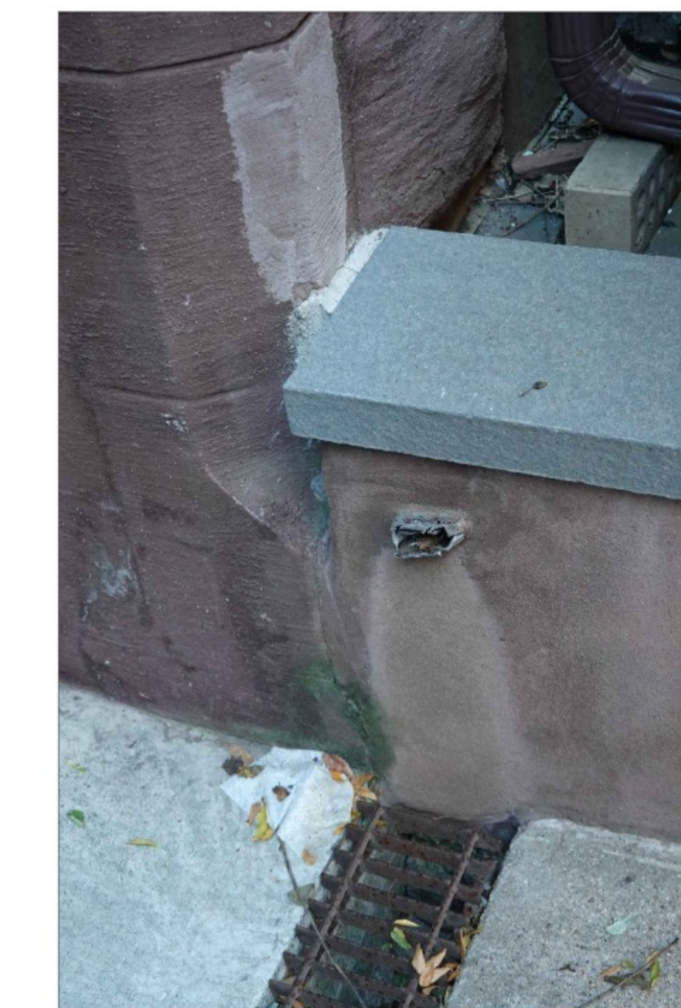
DRAINAGE CONDITION @ DRIVEWAY MKCA RECORDS 20
