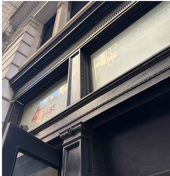
CLOSE UP IMAGE OF WOOD PILASTER TO HEADER CONNECTION AT SERVICE ENTRY
