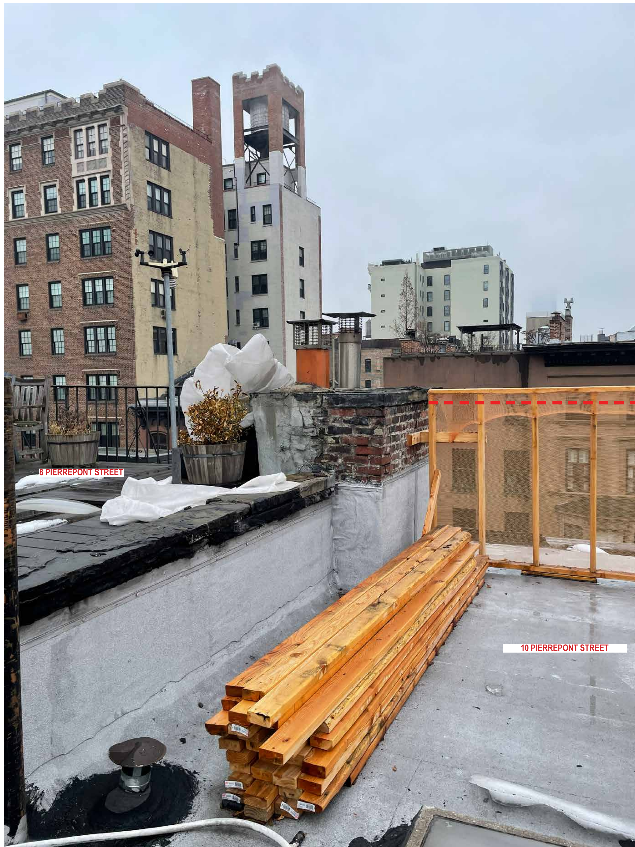
GUARDRAIL ALIGNMENT WITH 8 PIERREPONT
