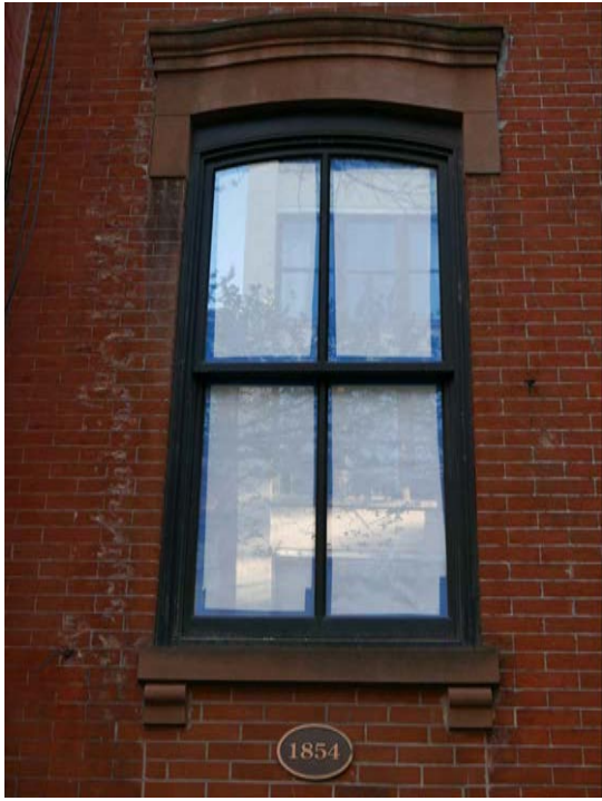
3 EXISTING PARLOR-LEVEL (1ST FLOOR) WINDOW ; NO BRICKMOLD, TYPICAL
