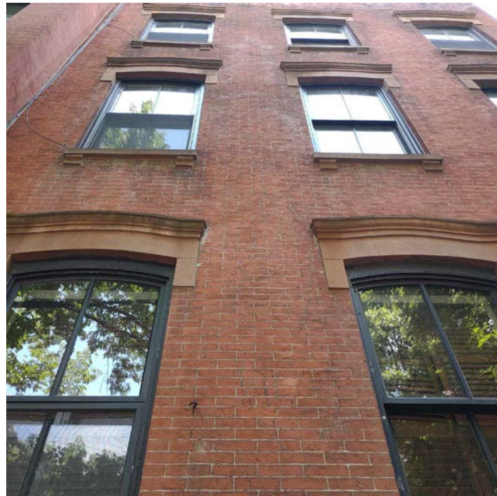
4 PHOTO SHOWING ABSENSE OF BRICKMOLD ON UPPER FLOORS
