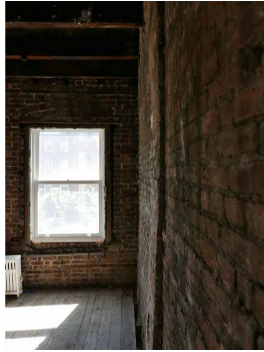
2 INTERIOR OF SOUTHERN END OF 3RD FLOOR WEST WALL, RAKING VIEW FACING SOUTH
