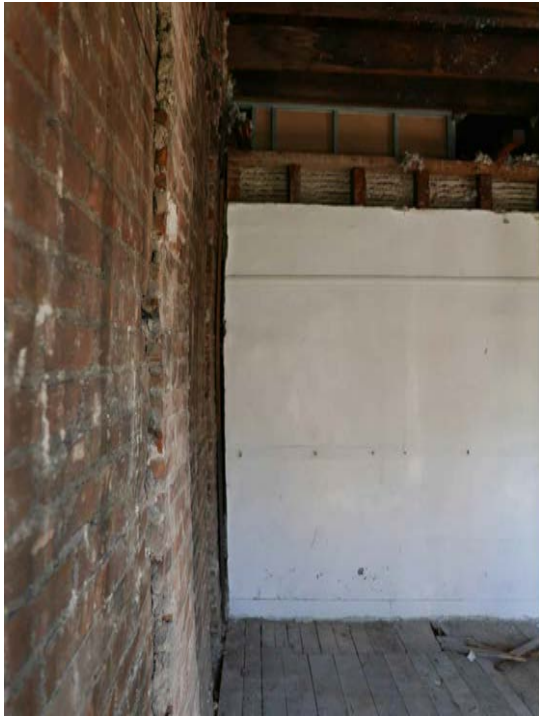
1 INTERIOR OF SOUTHERN END OF 3RD FLOOR WEST WALL, RAKING VIEW FACING NORTH
