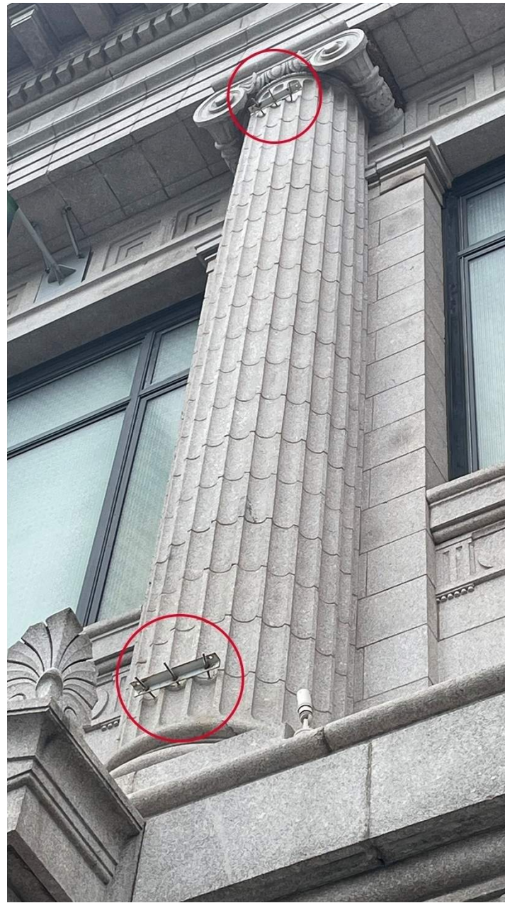
EXISTING BRACKET AT CENTER COLUMN TO REMAIN
