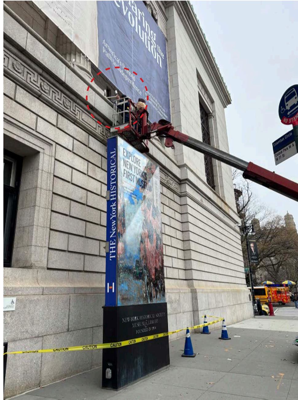
FIXTURE VISIBILITY LOOKING AT THE NORTH END OF THE COLONNADE AT CENTRAL PARK WEST FACADE
