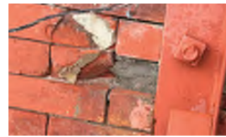
4. MISSING/ DAMAGED BRICK
