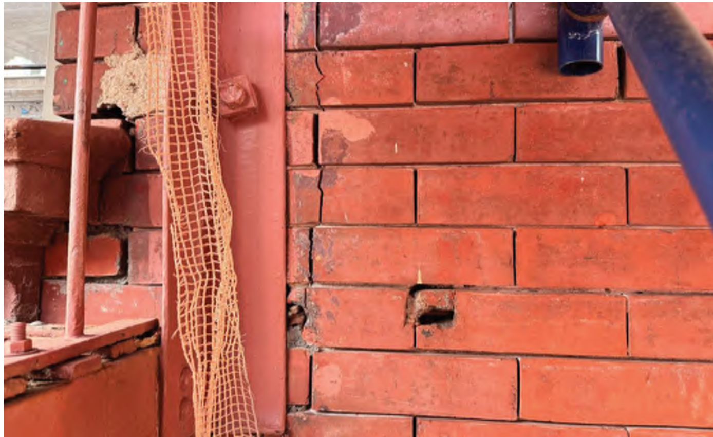
5 Vertical Brick Crack
