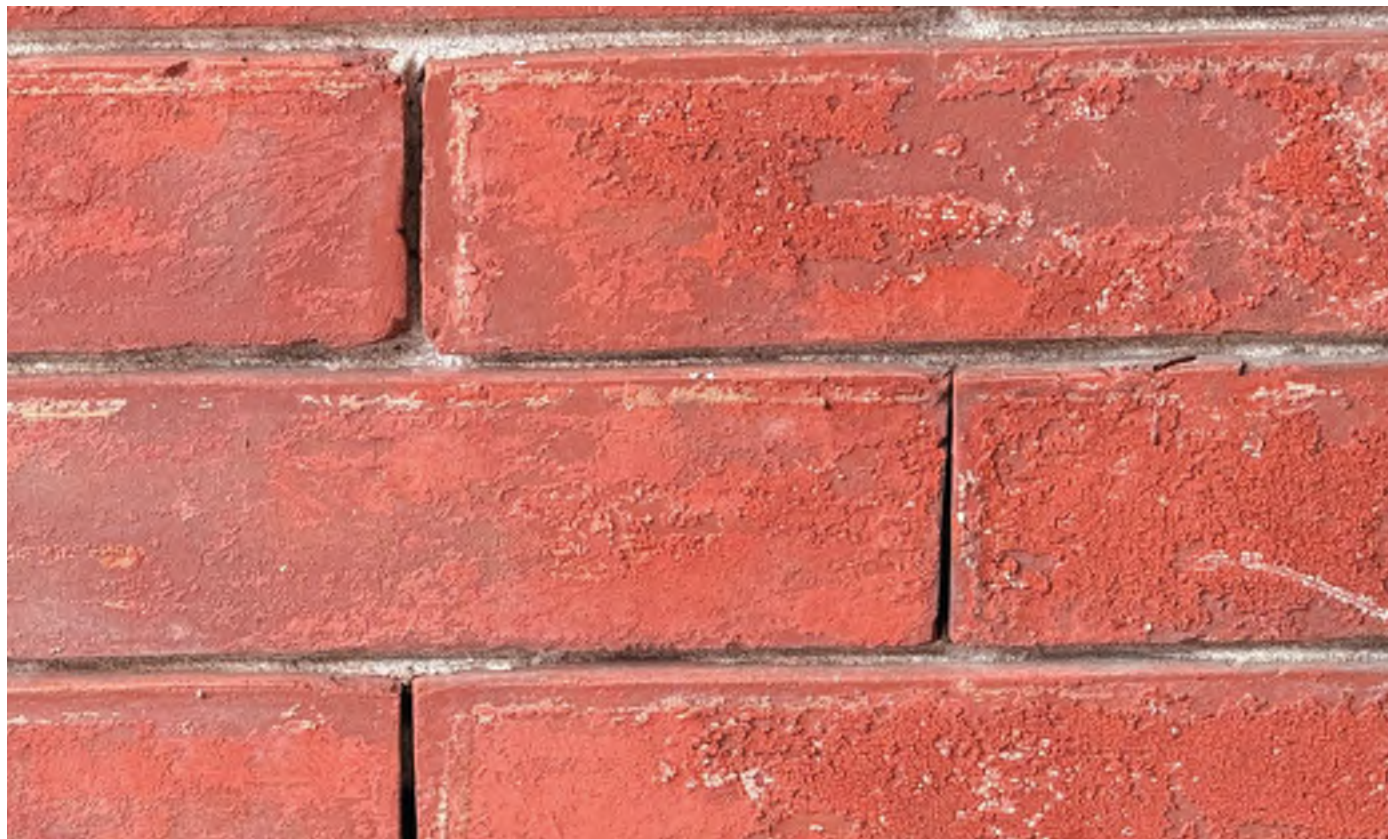
7 Former Coating Damage
