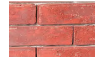
7. FORMER COATING DAMAGE
