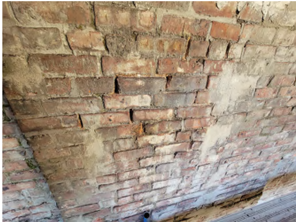
DEGRADATION OF FACADE BRICK (VISIBLE FROM SCAFFOLD)
