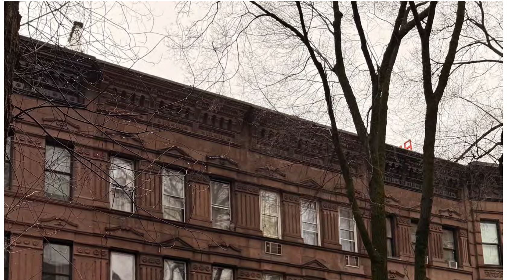
K - Wide angle View from 25 W 95th St. show flue mockup and neighboring flue
