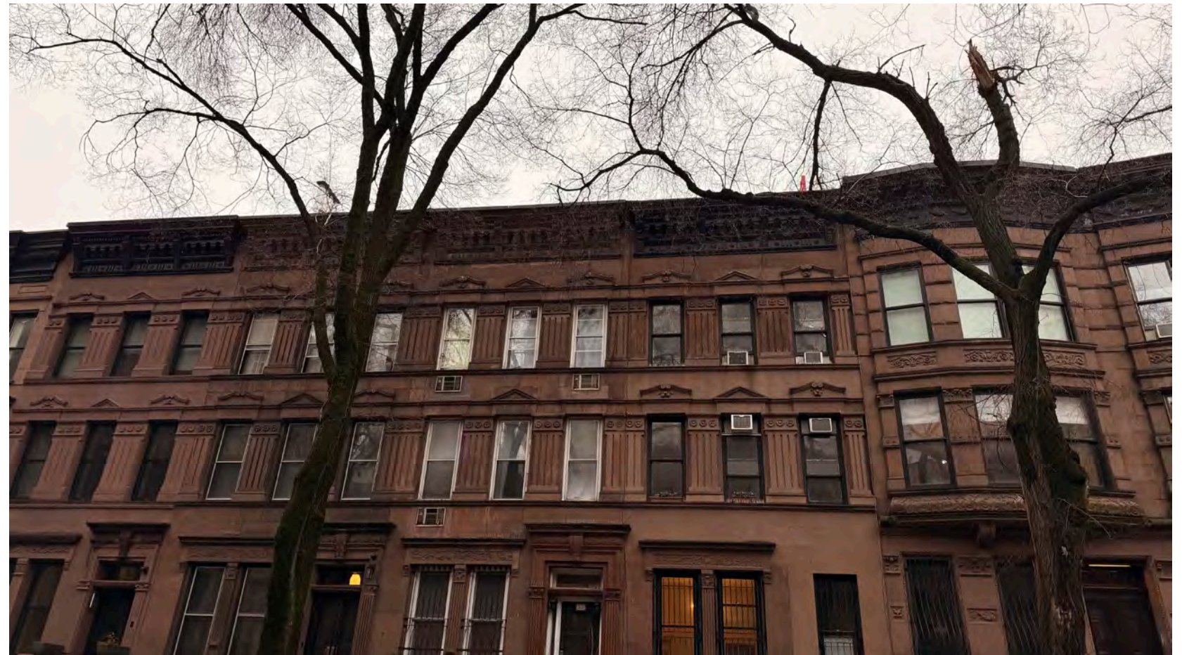
I - Wide angle View from 33 W 95th St. show flue mockup and neighboring flue
