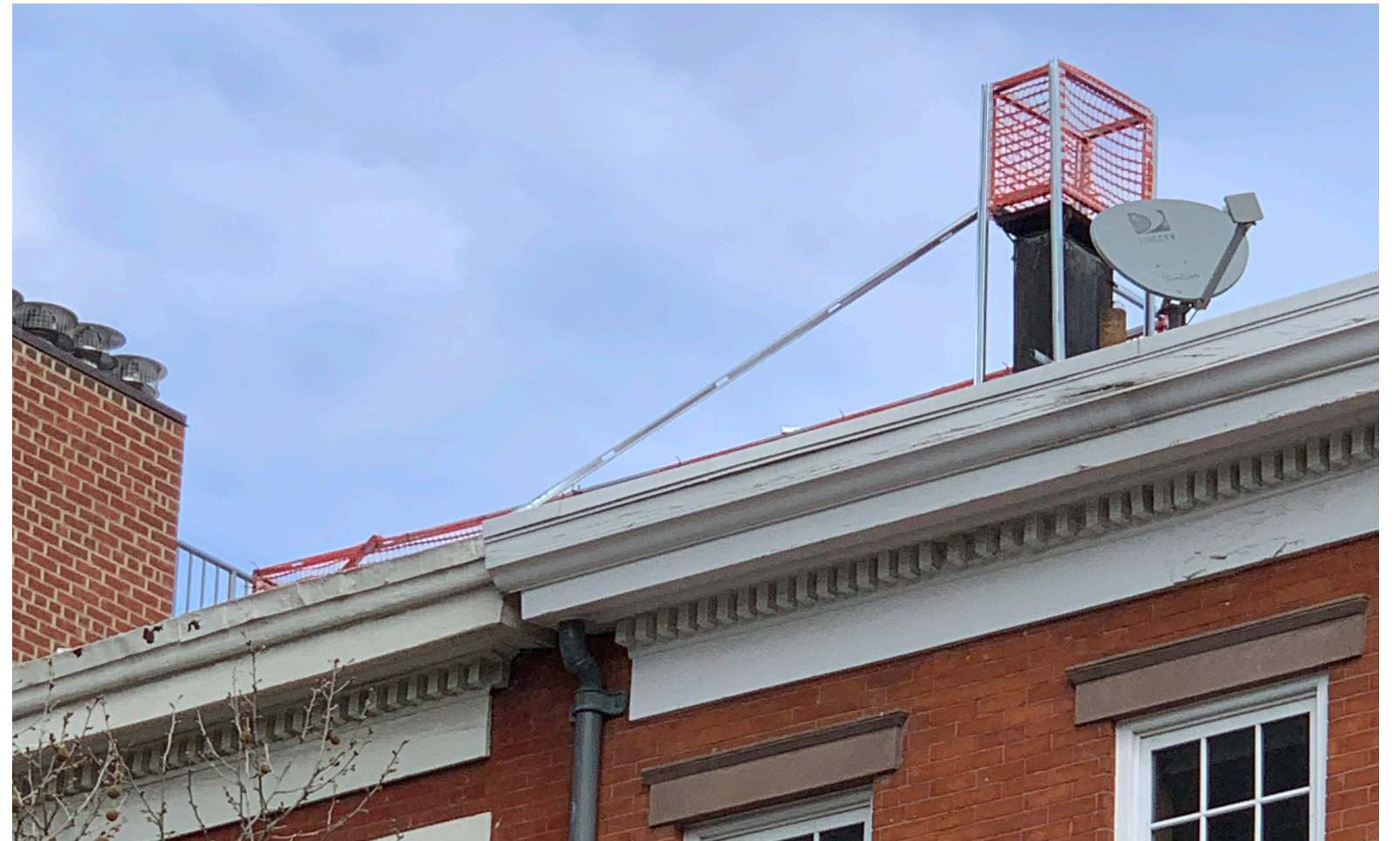
Detail view from west across Washington Street, chimney extension is visible, penthouse fascia is minimally visible
