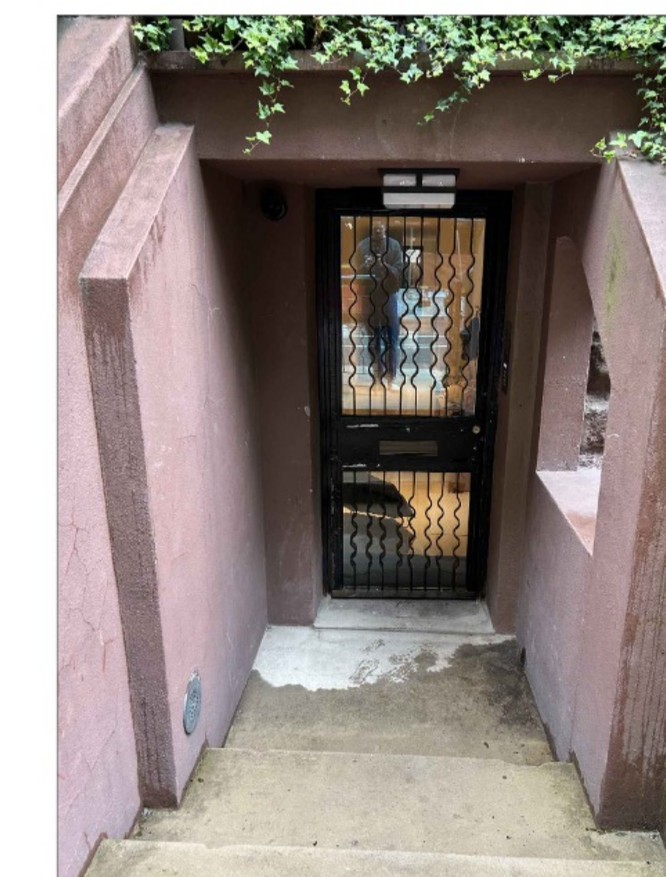
CURRENT WATER ISSUES @ AREAWAY MKCA RECORDS 10
