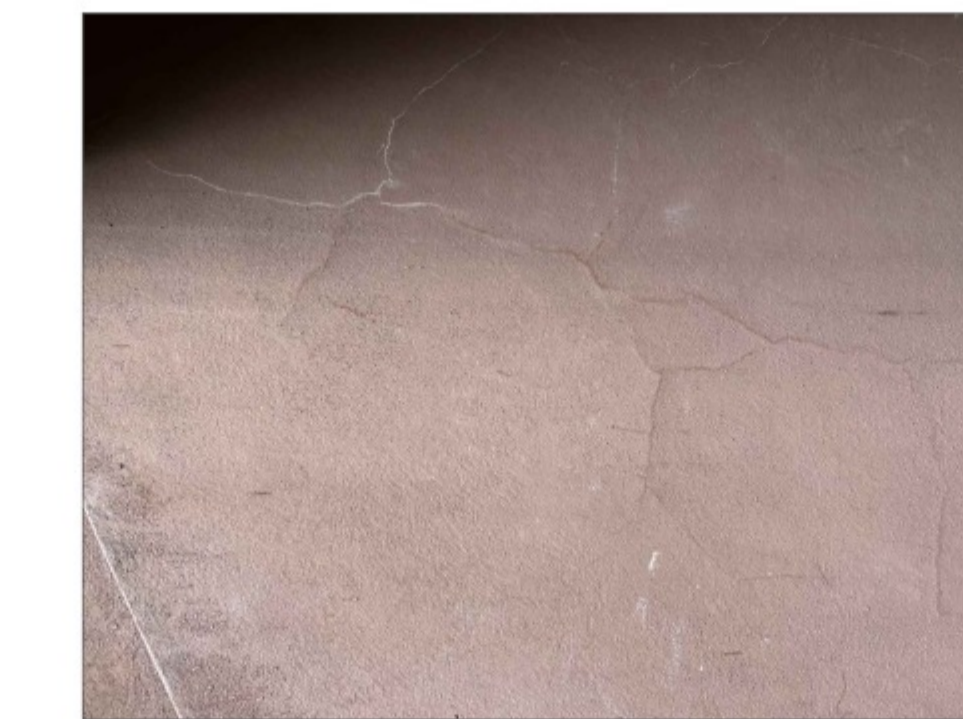
DAMAGED PARTS THROUGHOUT THE FACADE MKCA RECORDS 30
