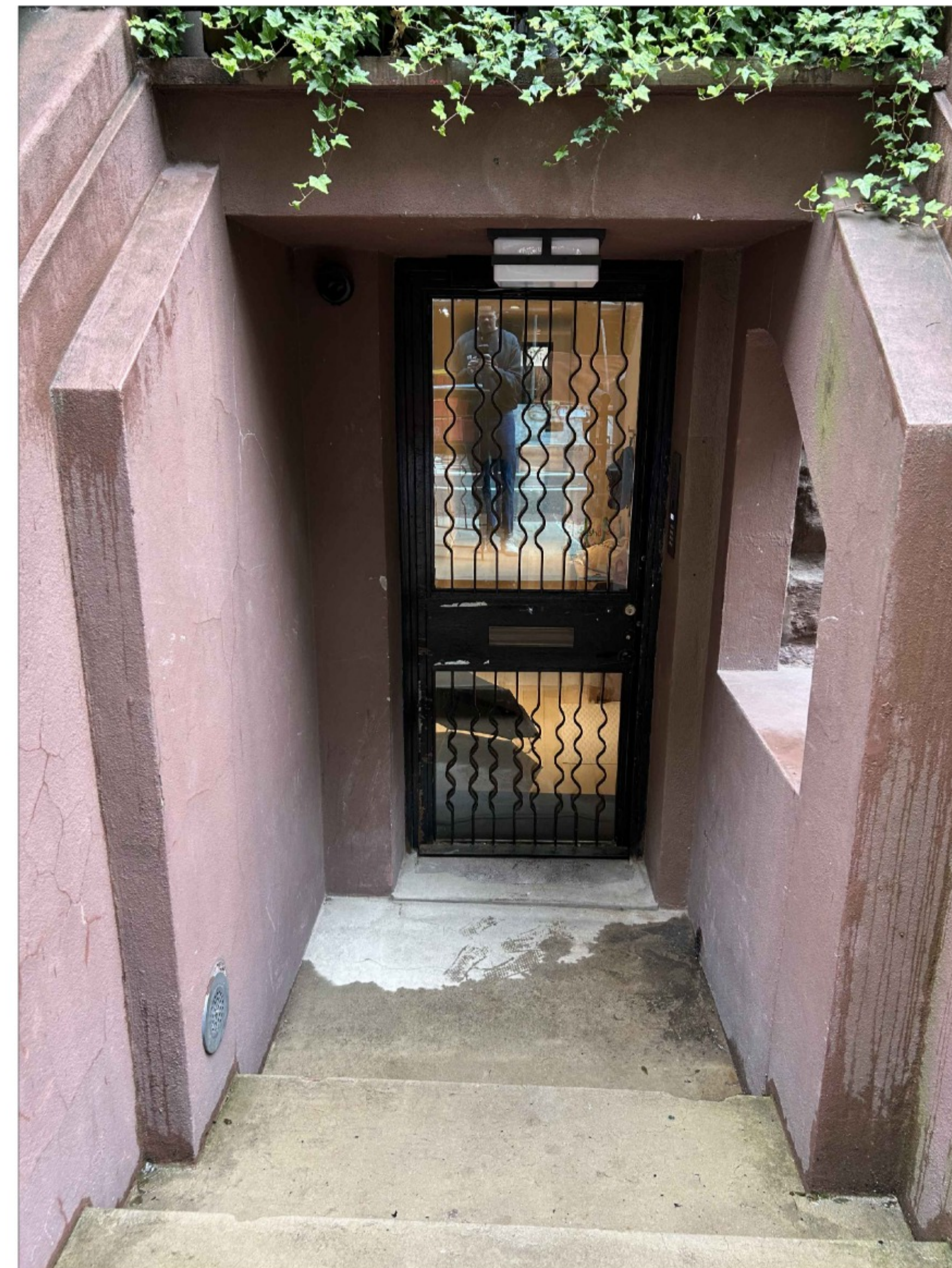
EXISTING AREAWAY LIGHT
