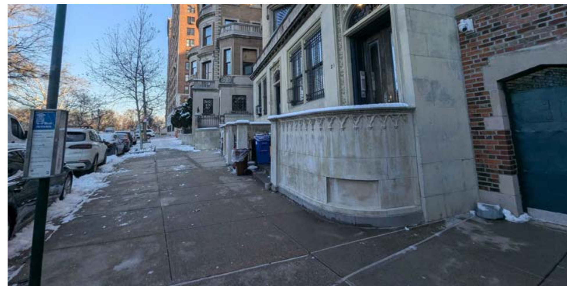
FENCE AND FRONT YARD PROTRUDING ON SIDEWALK
