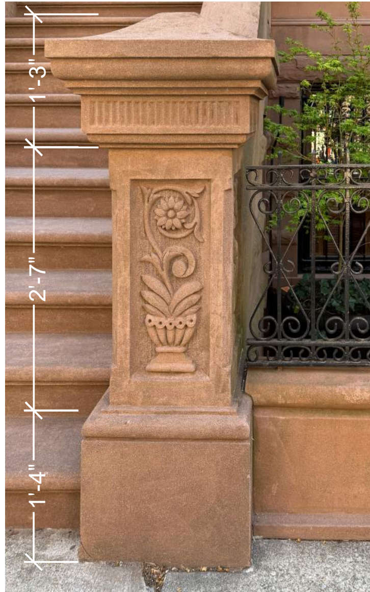
DETAILS OF POST AND RAILING TO MATCH THAT OF 160 WEST 88TH ST
