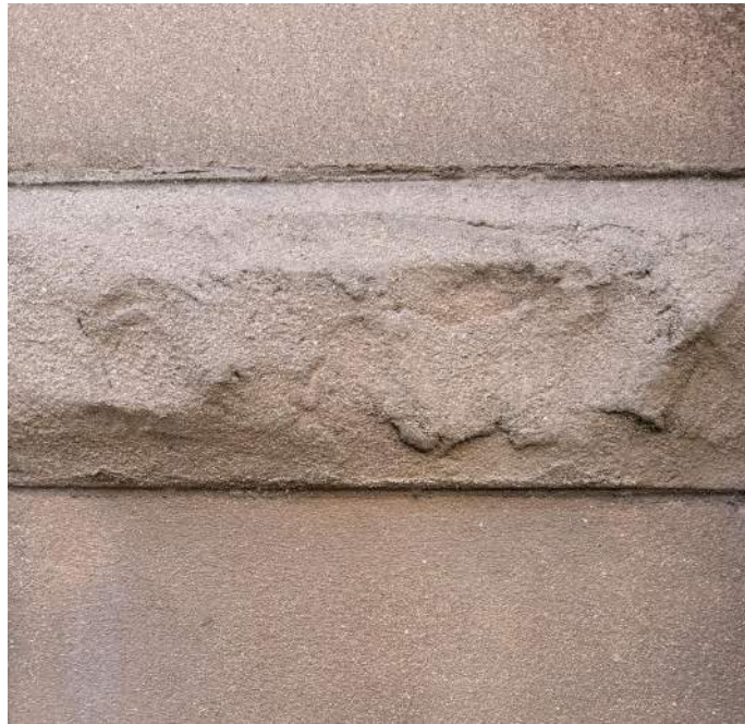
REFERENCE PHOTO OF EXISTING BROWNSTONE FINISH AND RUSTICATED BANDING AT BASEMENT LEVEL OF PRIMARY FACADE
