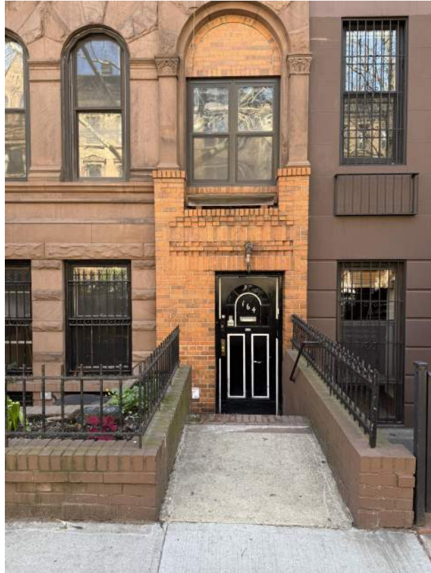
164 W 88TH STREET DOG-LEG STOOP REMOVED PRIOR TO LANDMARK DESIGNATION
