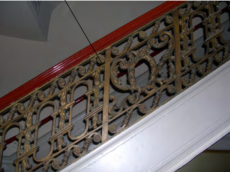
Pre-existing Designated Railing at HR Normal Exit Stair
