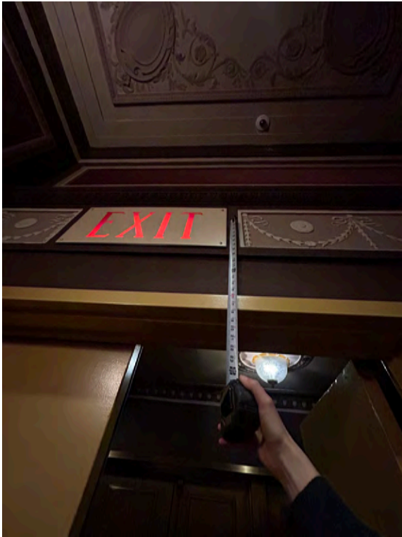
Current Photo of Header above House Right Doors
