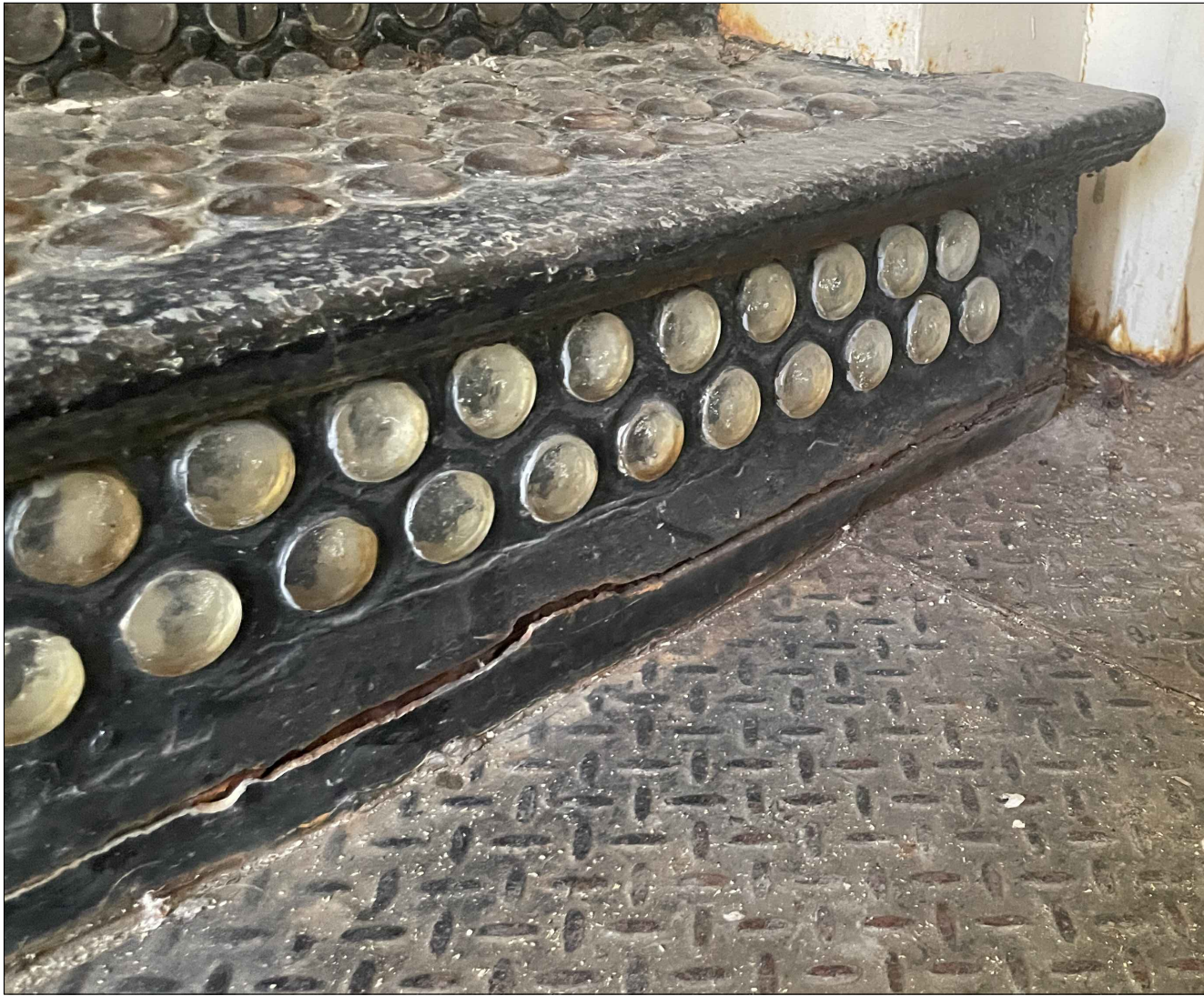
SOUTH STEPS (DAMAGE AS SEEN FROM ABOVE)
