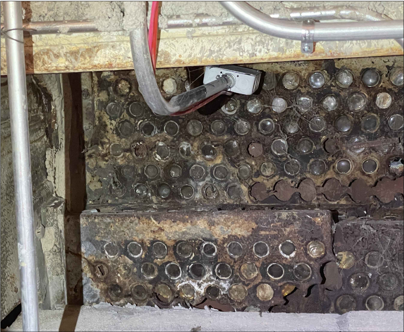
NORTH STEPS (DAMAGE AS SEEN FROM BELOW)
