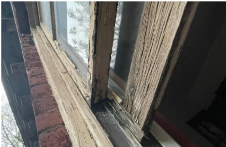
Severe Window Frame Deterioration
