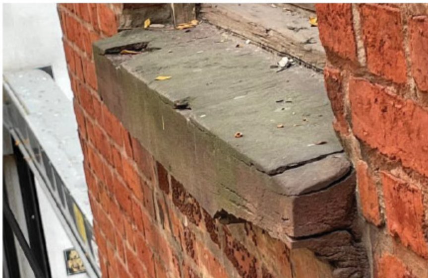
Stone Sill Deterioration
