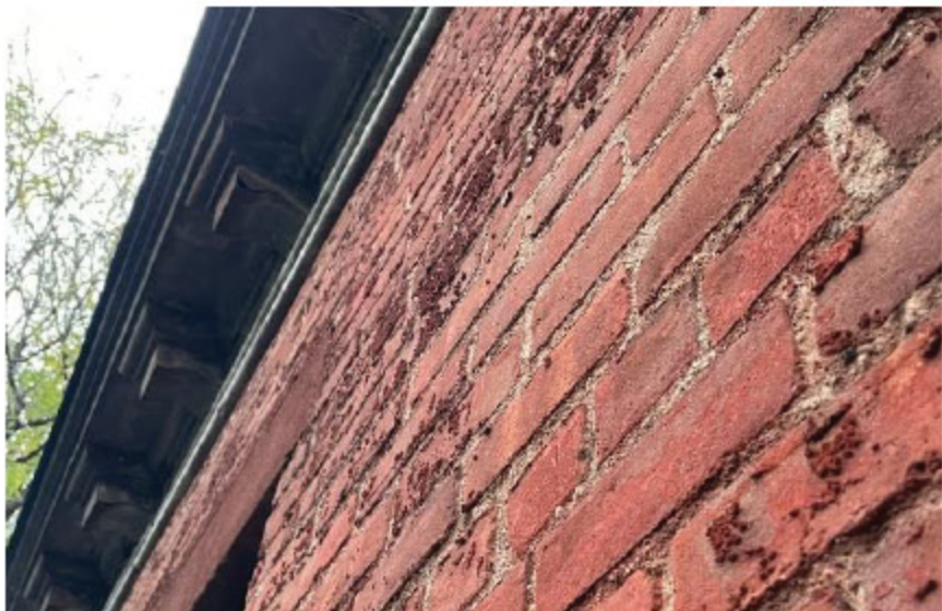
Flaking Paint Residue
