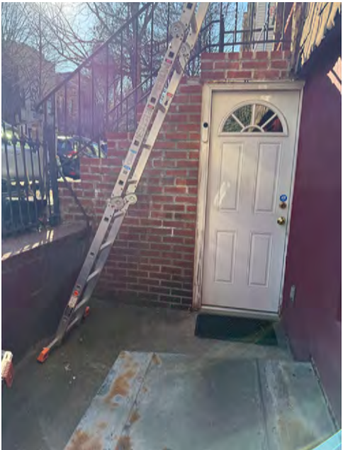
113 NOBLE STREET, EXISTING FRONT AREAWAY UNDERSTOOP DOOR
