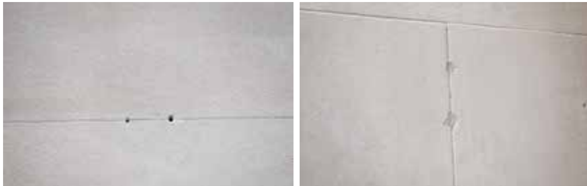
WALL DAMAGE & SUBSTANDARD REPAIR
