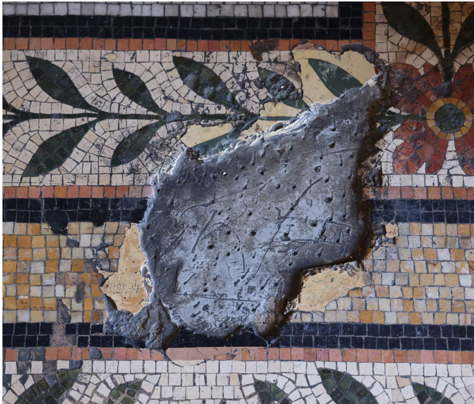
Damaged Exterior Mosaic
