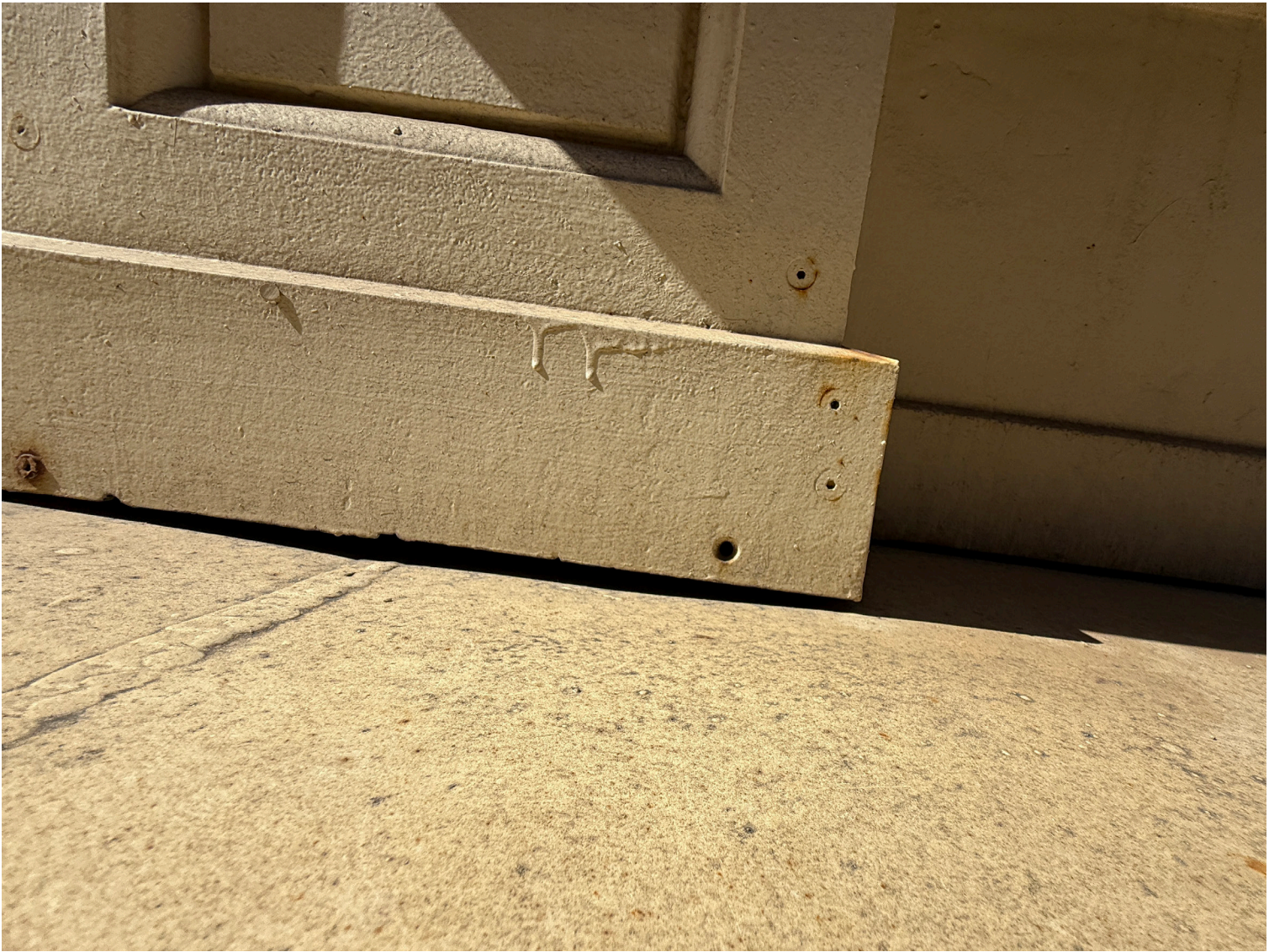
Replace all missing fasteners in kind.
