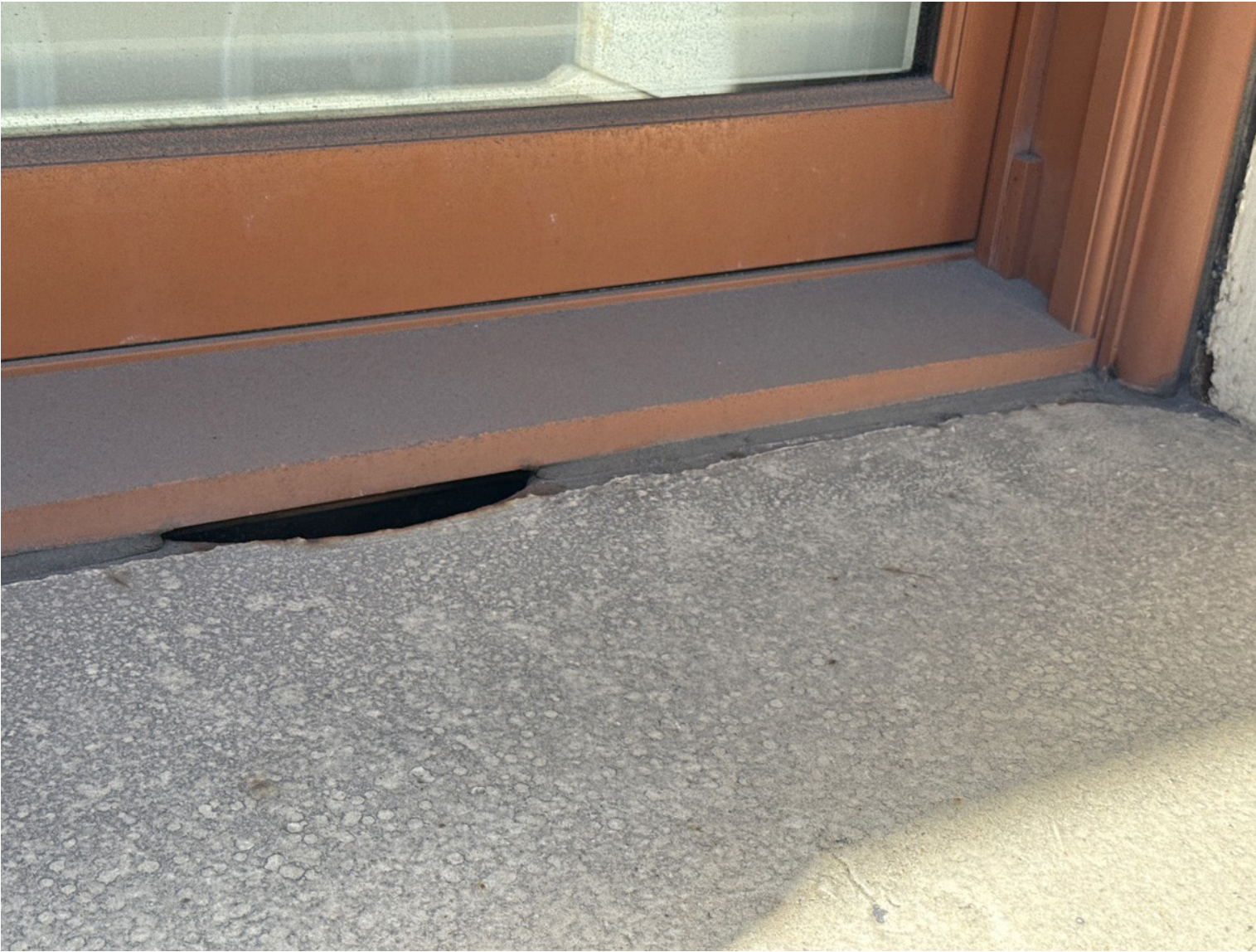
Replace missing window perimeter sealant
