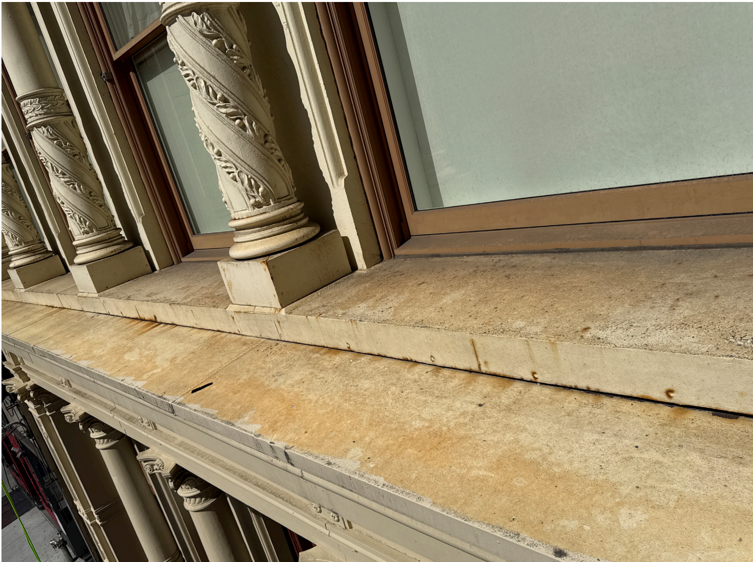
Scrape, prime and re-paint existing cast iron where there is evidence of corrosion.
