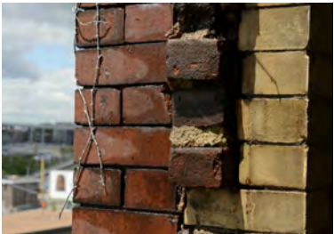
TYPICAL CONDITION OF WINDOW SURROUNDS REQUIRING PREPARATION FOR WINDOW INSTALLATION
