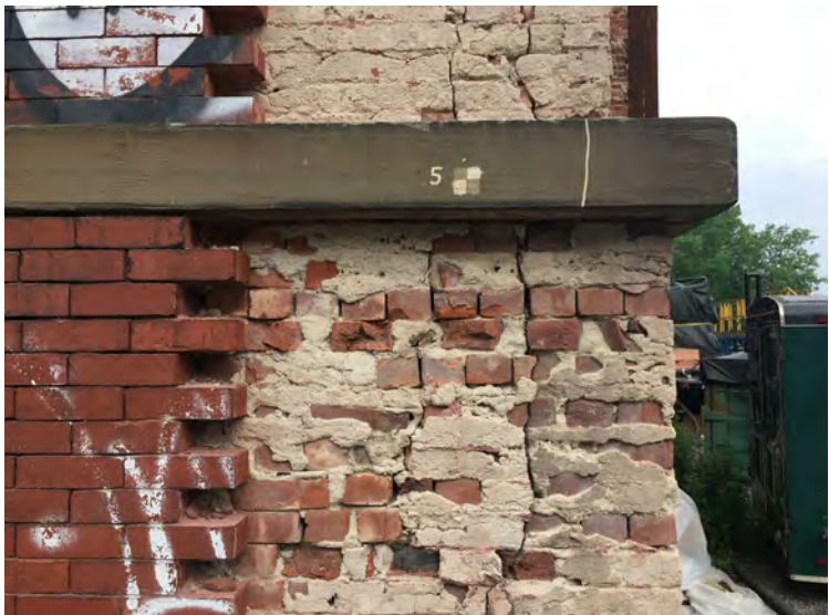
TYPICAL CONDITION OF FACEBRICK AND BACKUP REQUIRING CORNER RECONSTRUCTION
