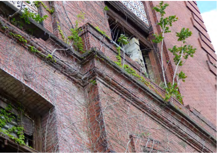
TYPICAL CONDITION OF BIOLOGICAL GROWTH TO BE REMOVED
