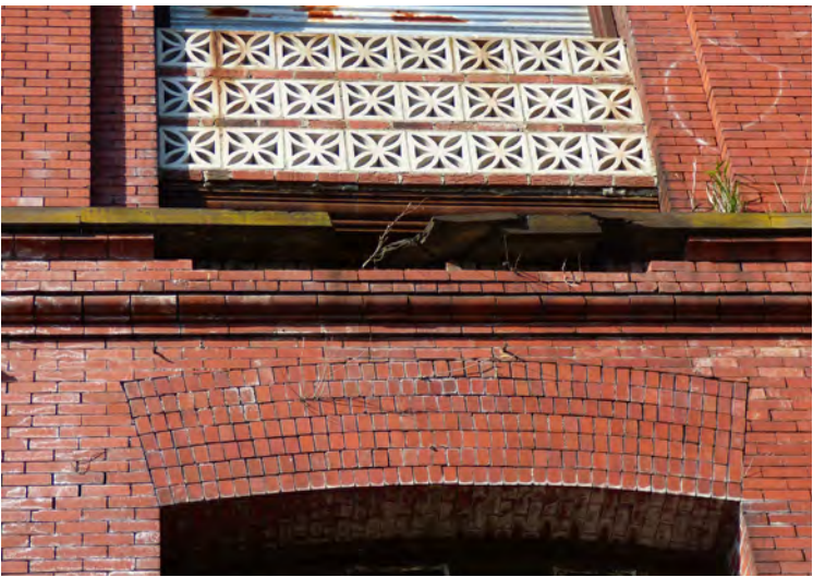
TYPICAL CONDITION OF BLUESTONE UNITS REQUIRING FULL OR PARTIAL REPLACEMENT
