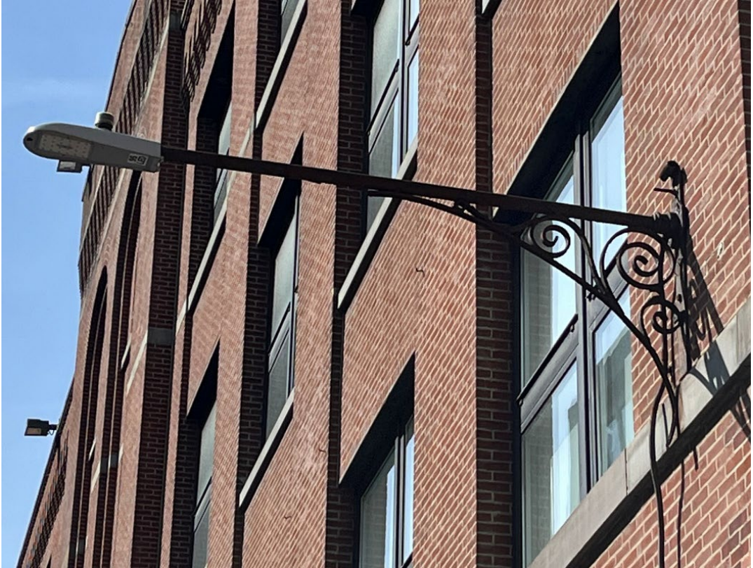
Existing historic metal bracket and non-historic luminaire. Exterior conduit and non-historic luminaire to be removed (2 typical).
