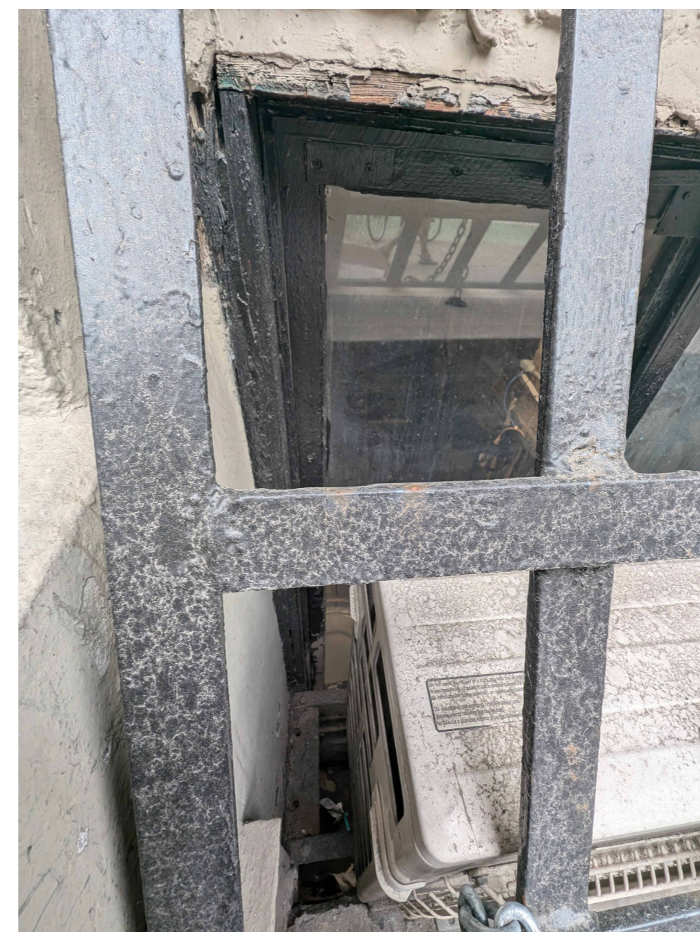
CONDITION OF THE EXISTING CELLAR WINDOW TO BE REMOVED
