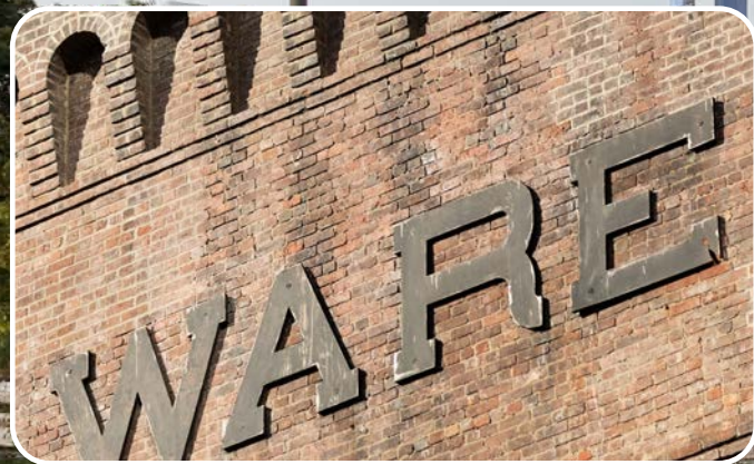
EXISTING SIGNAGE AT 11TH AVENUE 1 1/2" DEEP CAST METAL LETTERS W/ 1" DIAMETER SCREWS
