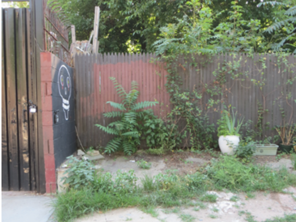
211 WAVERLY AVENUE SIDE WALL & 221 WAVERLY AVE FENCE CONDITION
