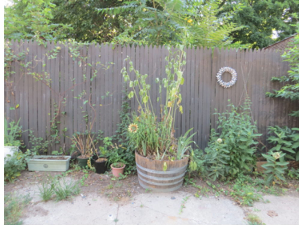
221 & 223 WAVERLY AVE FENCE CONDITION
