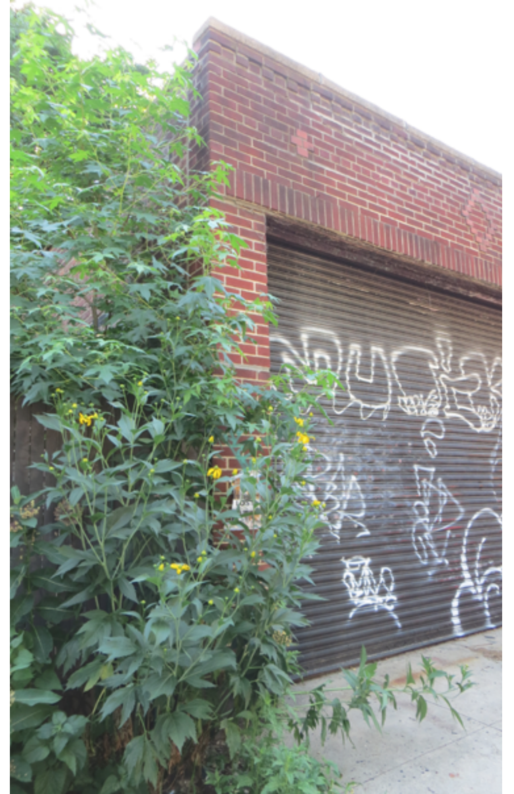
223 WAVERLY AVE FENCE CONDITION & 225 WAVERLY AVENUE GARAGE CONDITION
