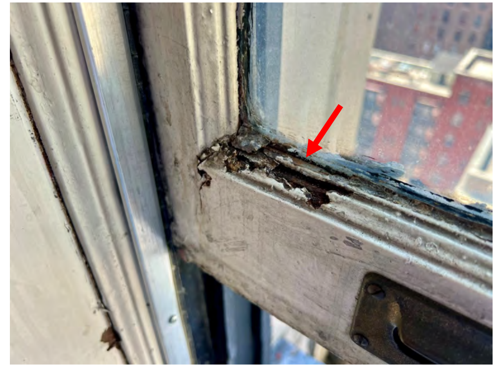
4. Interior- Note failure of sheet metal cladding/wood deterioration lower sash
