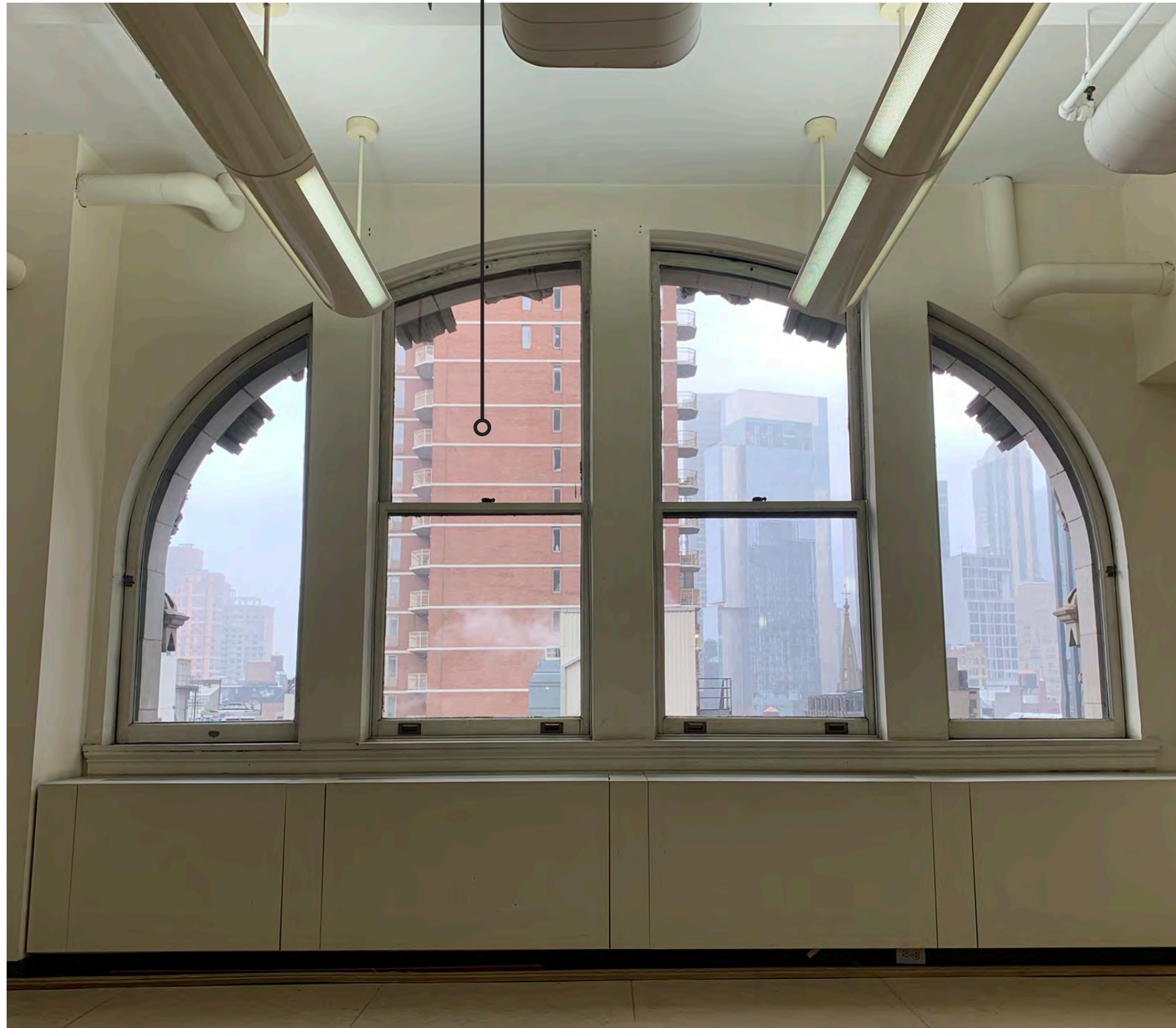
Replacement Window: Inswing casement lower lite with arched fixed lite on top to match existing profile
