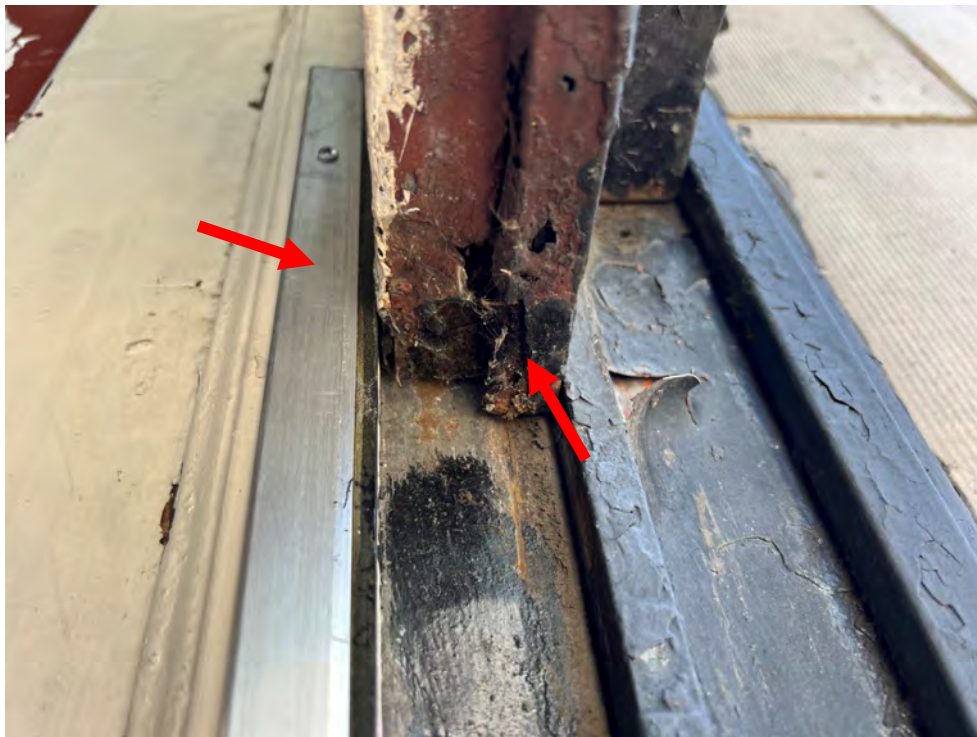
5. Bottom sash- Note deteriorated sheet metal cladding/added weatherstripping
