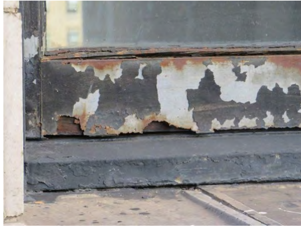
2. Exterior- Note sheet metal cladding failure
