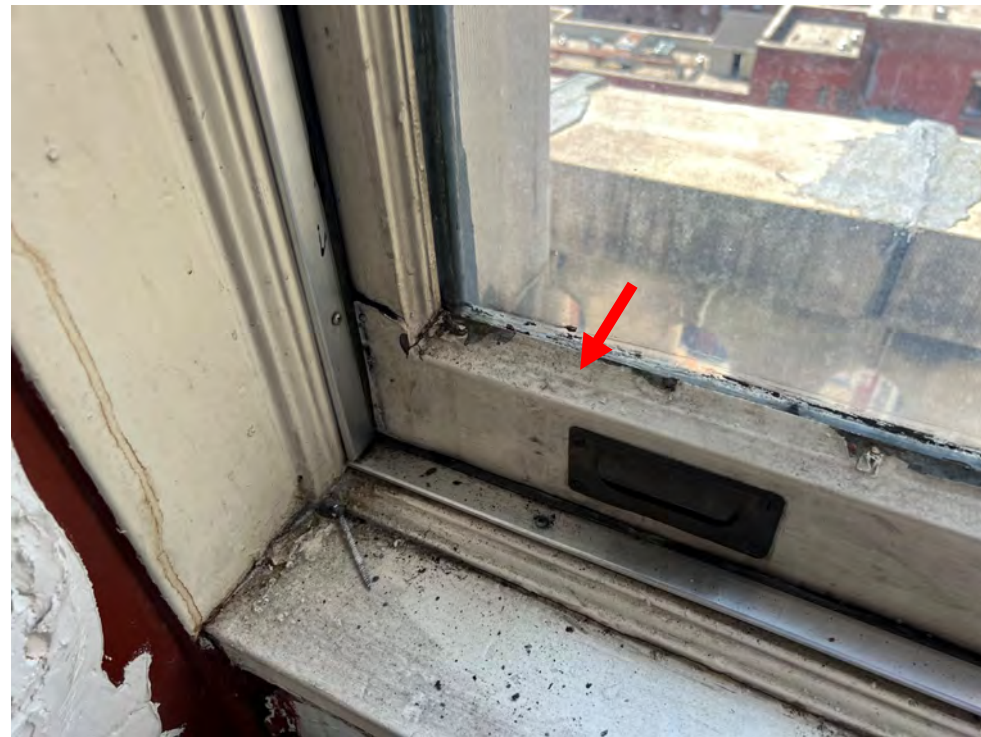
6. Bottom sash- Typical sash repair with sheet metal. Poor condition
