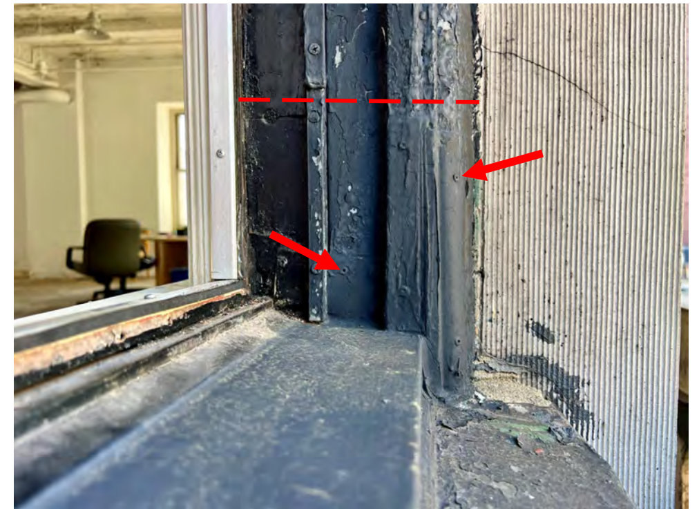
9. Jamb- Typical lower jamb repair (below dashed line) with new sheet metal cladding, pop-riveted to substrate. Poor condition. Limits sash operation.
