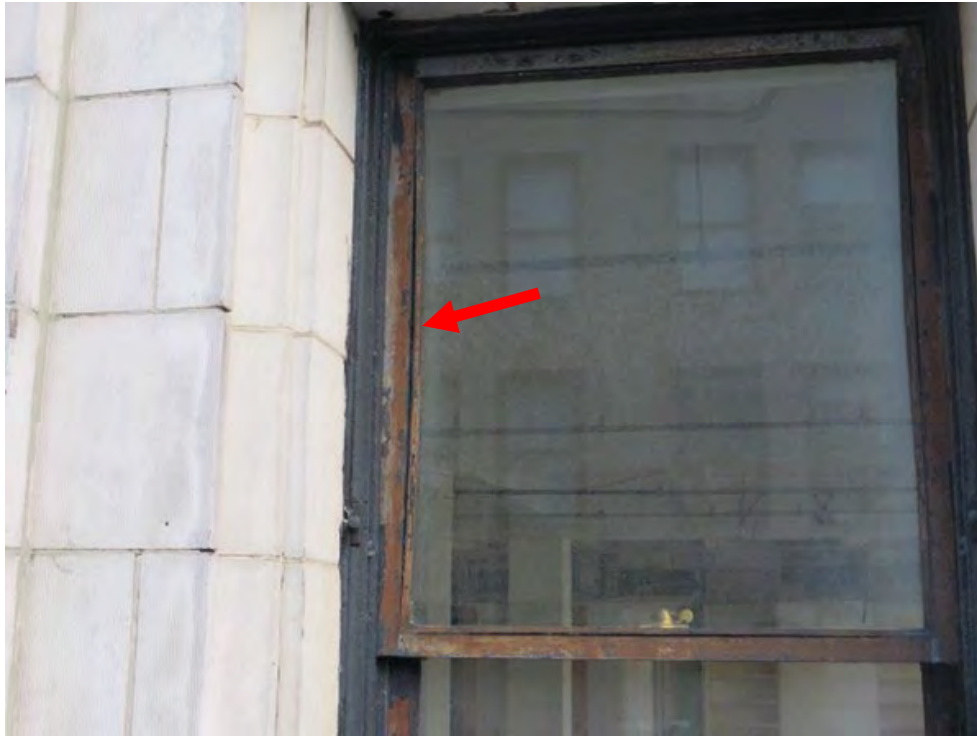
1. Exterior – Note loss of galvanizing, rust and failing glass stop.
