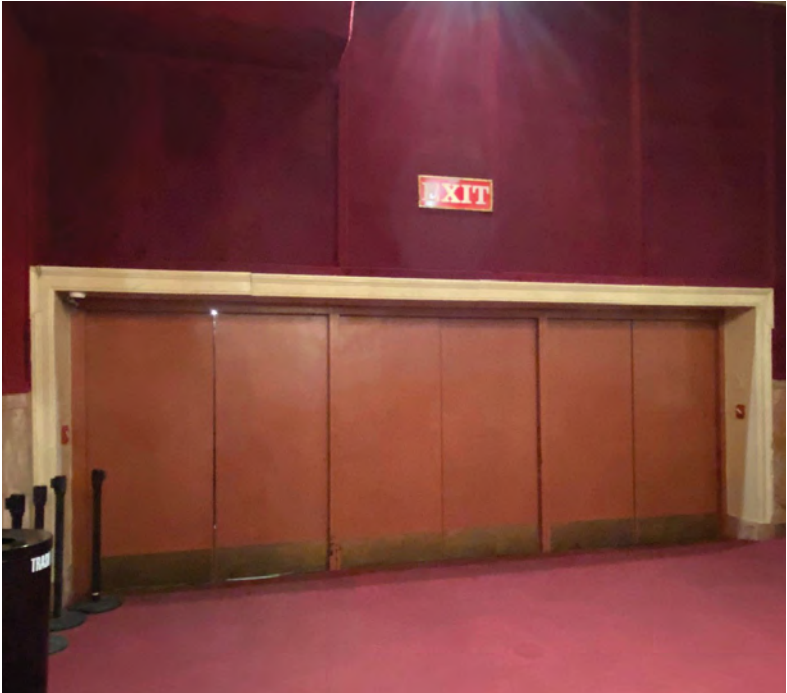
EXISTING EXIT SIGN AT 126TH ST EXIT, NOT CODE COMPLIANT, REPLACED WITH EX-01 EXIT SIGN
