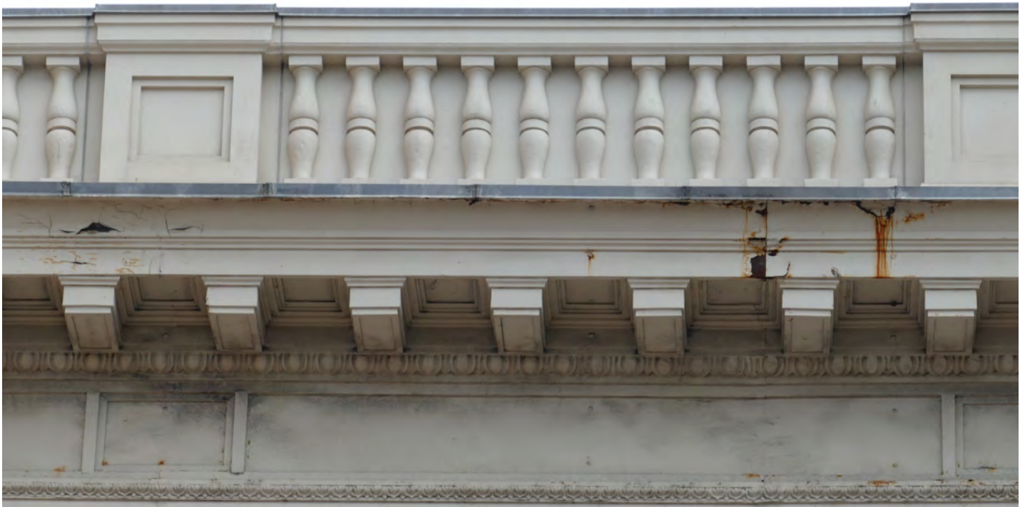
METAL DETERIORATION AT CORNICE
