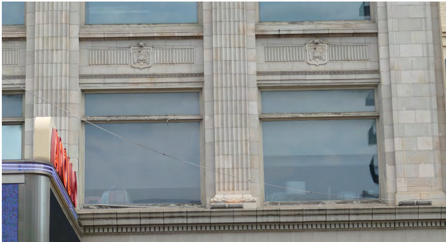
PAINT FAILURE AND WOOD DETERIORATION AT FRONT FACADE WINDOWS
