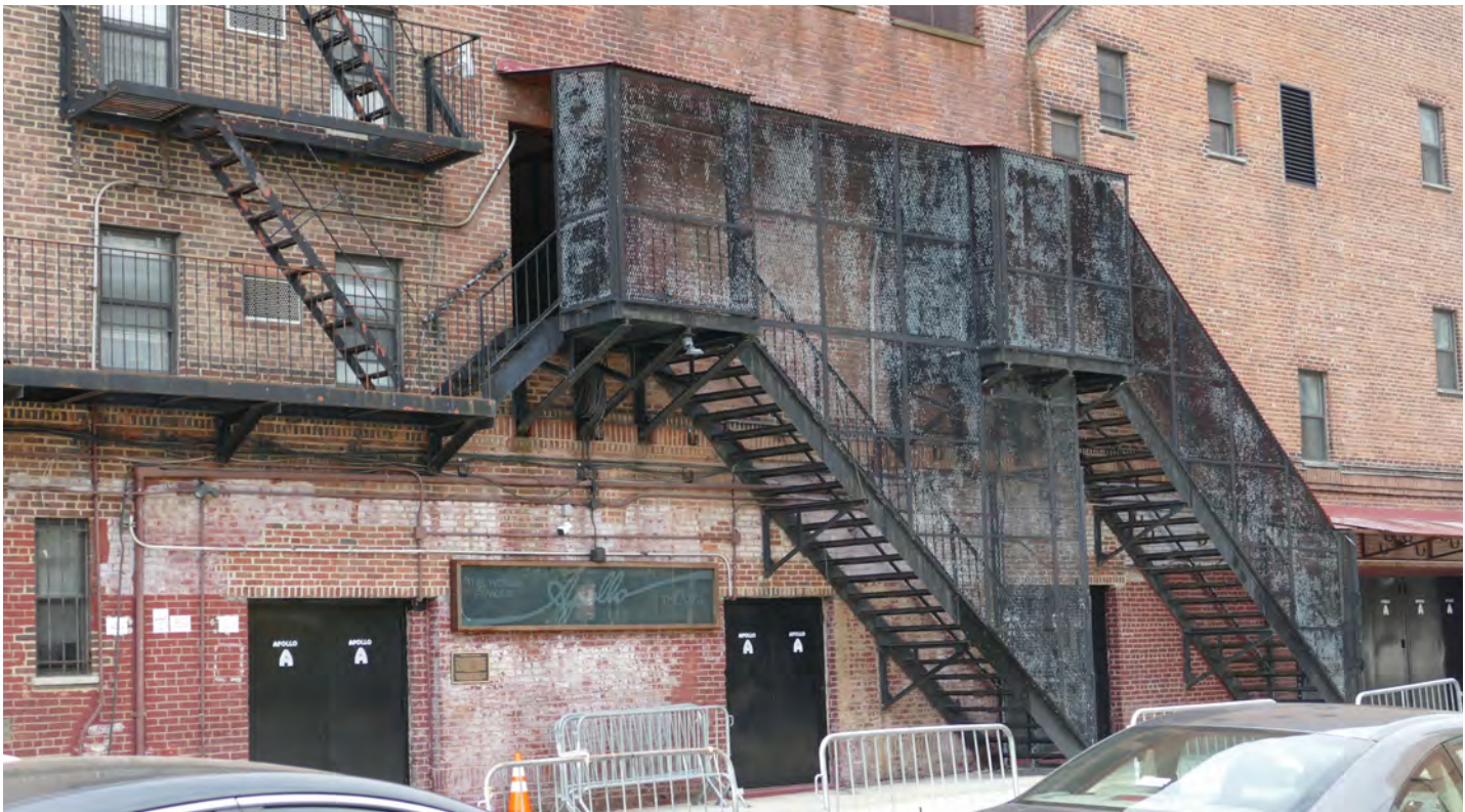
PAINT FAILURE AT WEST 126TH STREET FACADE
