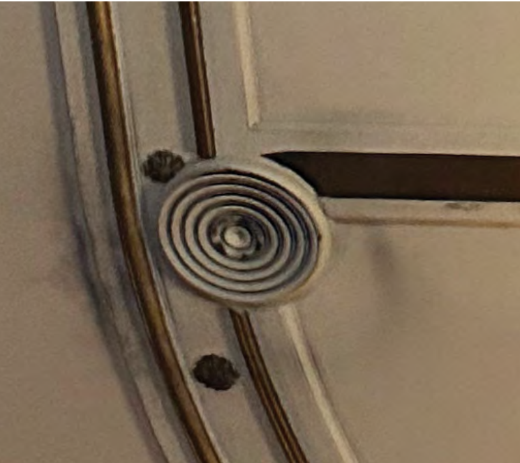
EXISTING PAINTED ROUND DIFFUSERS AT AUDITORIUM CEILING
