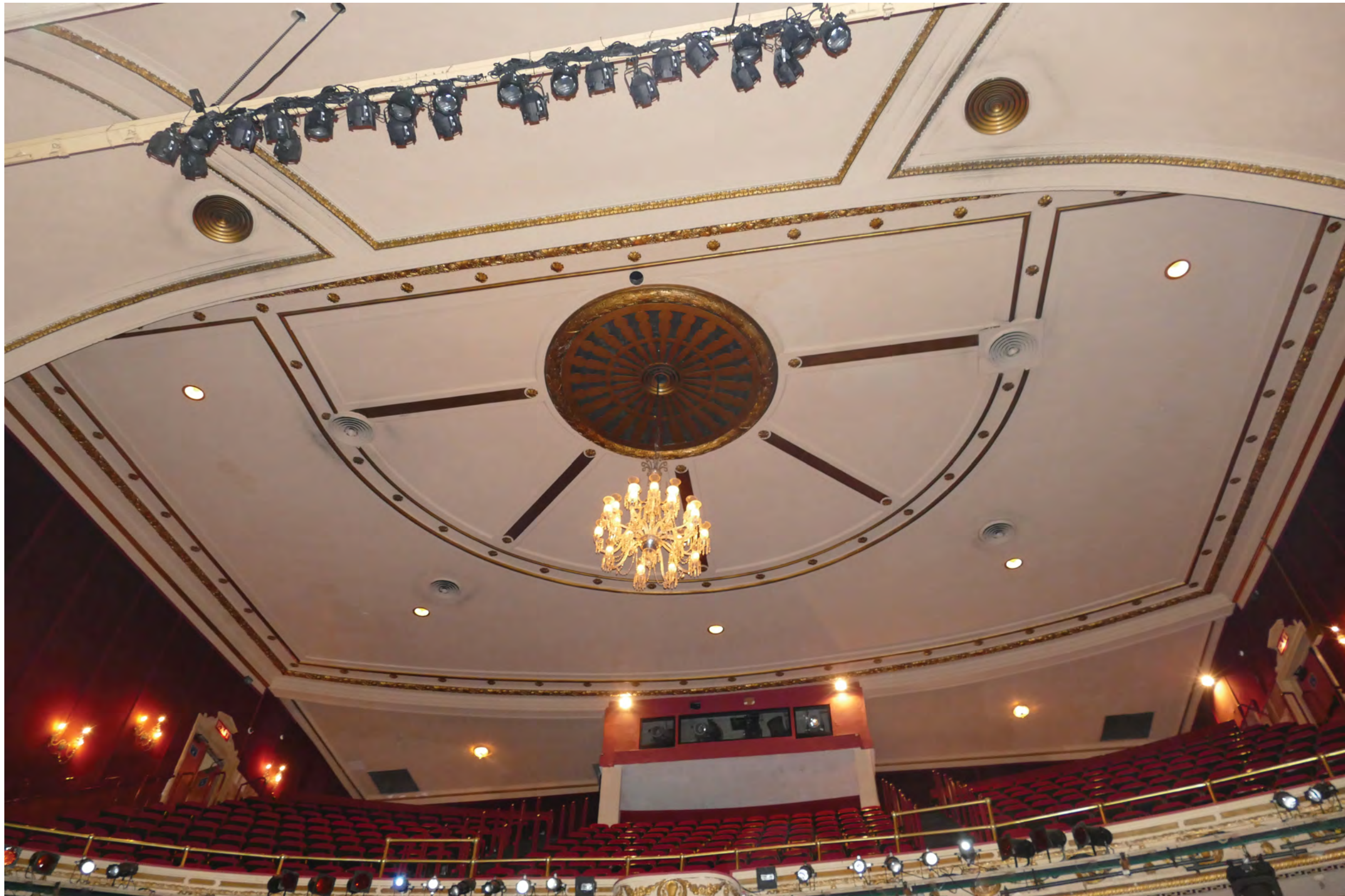
EXISTING AUDITORIUM CEILING CONDITIONS
