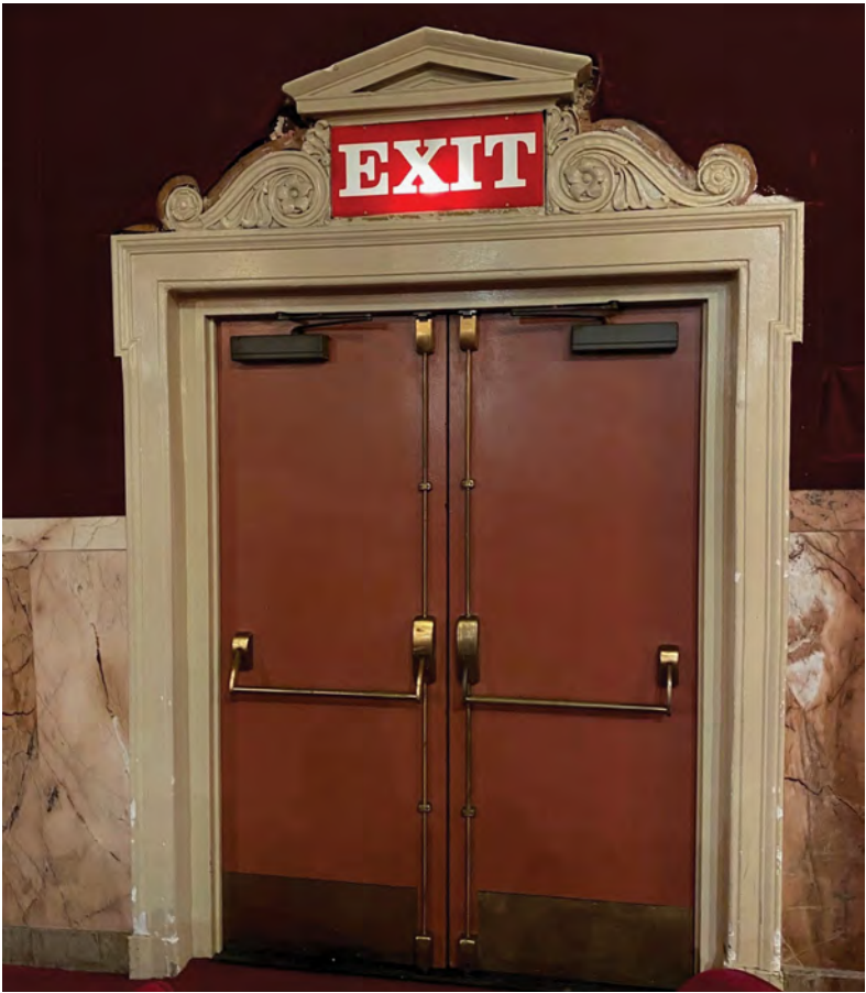
EXISTING EXIT SIGN AT ORCHESTRA & BALCONY LEVEL HISTORIC EXIT TO STAIRS, NOT CODE COMPLIANT, REPLACED WITH EX-02 EXIT SIGN
