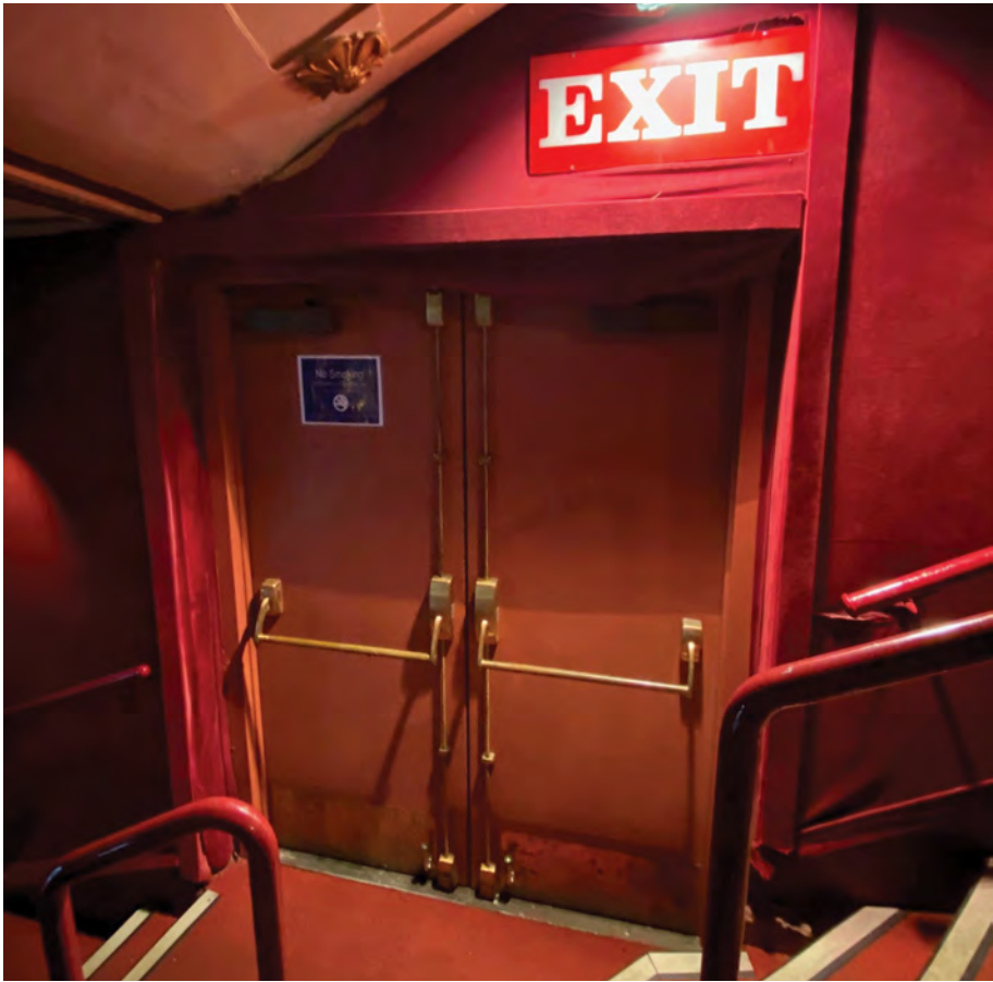
EXISTING EXIT SIGN AT MEZZANINE TO STAIRS, NOT CODE COMPLIANT, REPLACED WITH EX-01 EXIT SIGN
