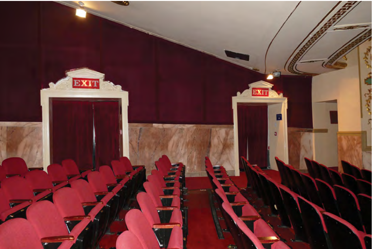
VIEW D - LOOKING NORTH, MARBLE WAINSCOT IS NON-HISTORIC, AS IS FABRIC CLADDING ABOVE. EXIT SIGNS DO NOT MEET CURRENT CODE.
