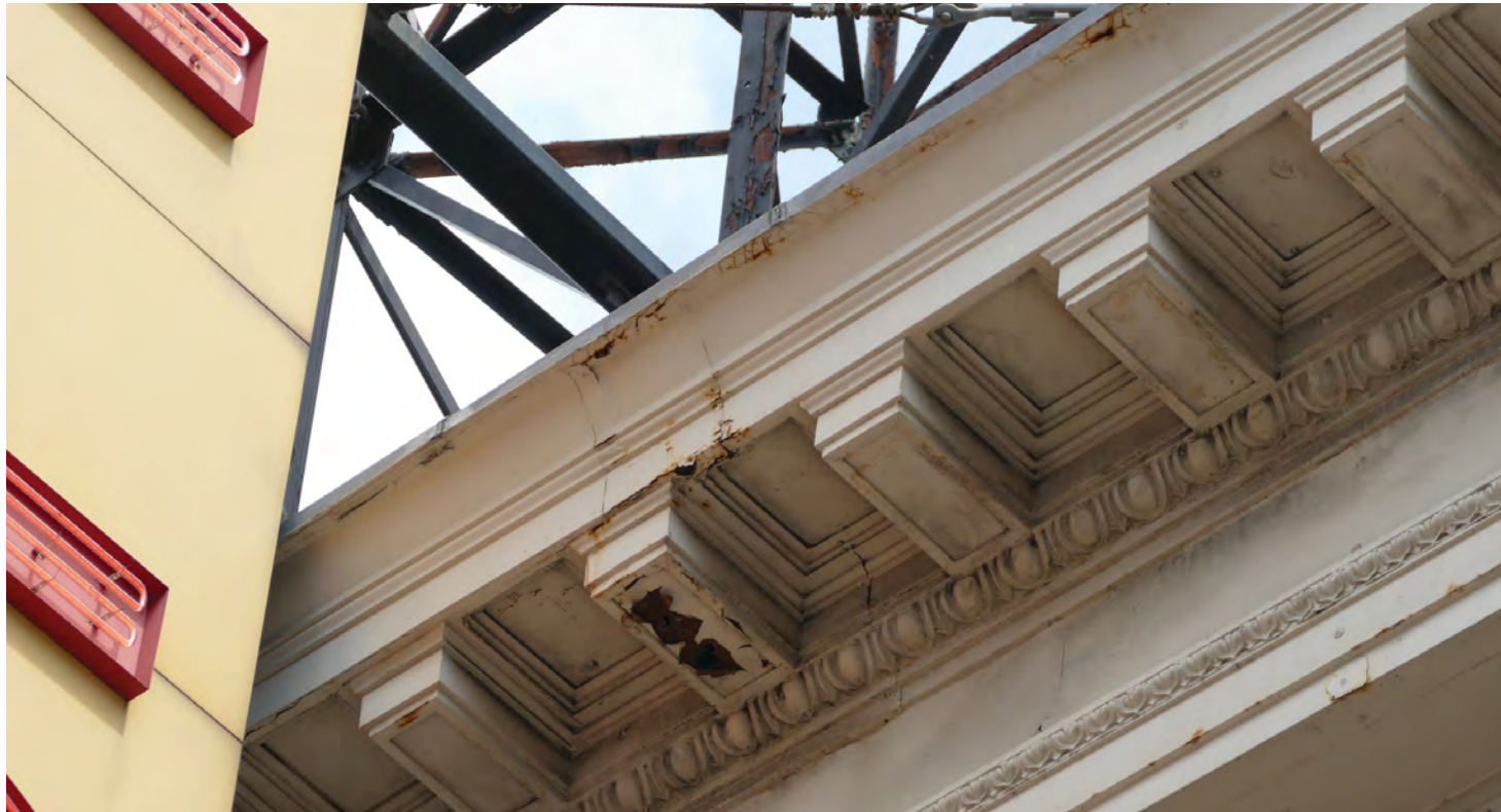
PAINT FAILURE AND RUSTING AT METAL CORNICE AND STRUCTURE SUPPORTING BRACKET SIGN
