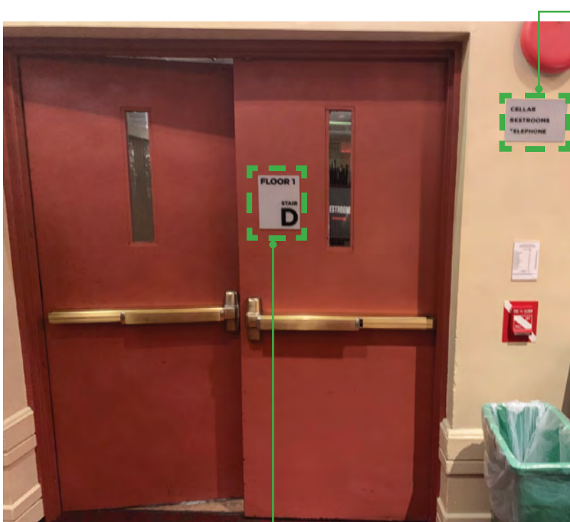
EXISTING ACCESSIBILITY SIGNAGE WITHOUT BRAILLE - NOT CODE COMPLIANT, INCORRECT LOCATION
