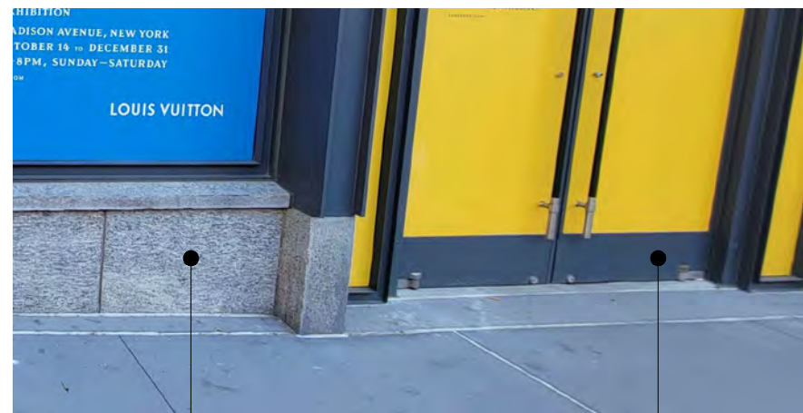
EXISTING GRANITE - WOOD CREEK GRANITE - THERMAL FINISH NEW INFILL TO MATCH EXISTING
