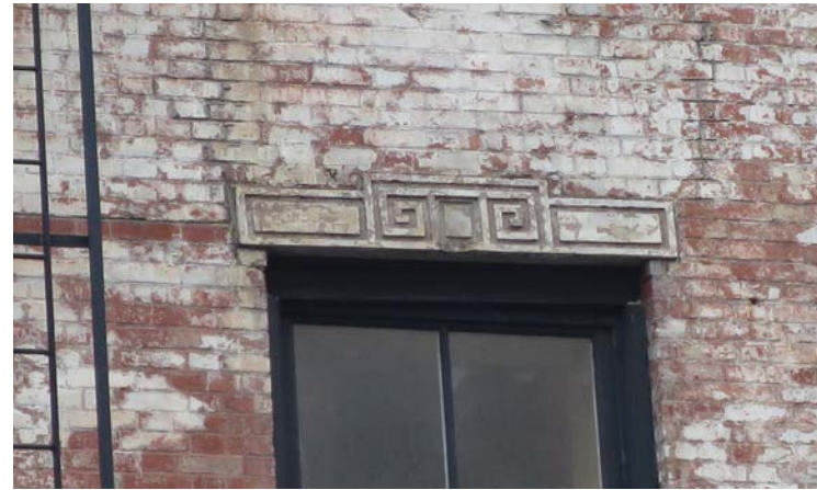
Window lintel at second floor. Painted brownstone with some minor damage.
