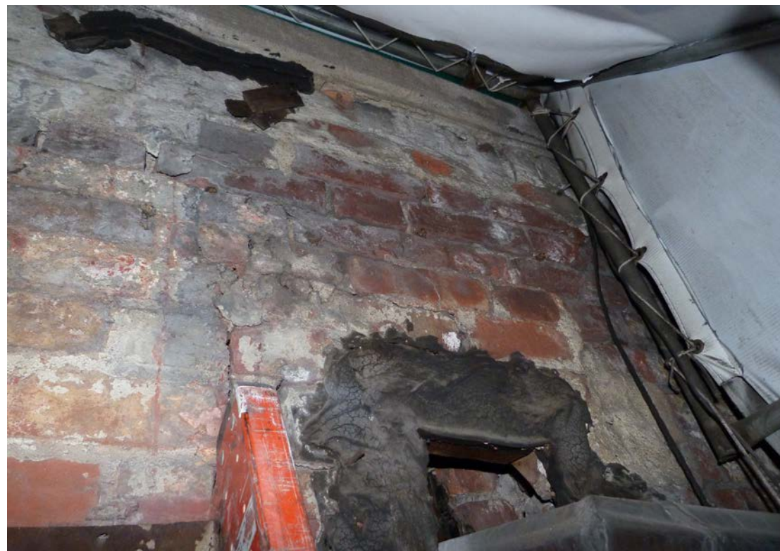
421 Broadway Typical brick condition at spandrel
