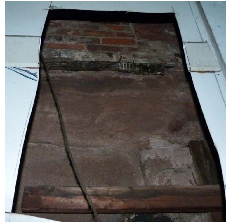
421 Broadway Brownstone stringcourse with two generations of brick above; brick has been coated
