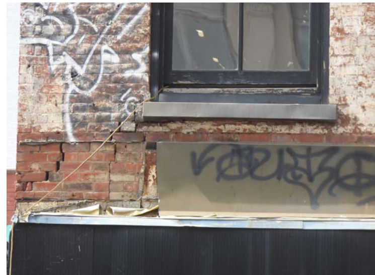
Brownstone window sills have non-historic aluminum caps. The brick facade is experiencing some step cracking. Graffiti exists at the second floor of the primary facade and along the southern side wall.
