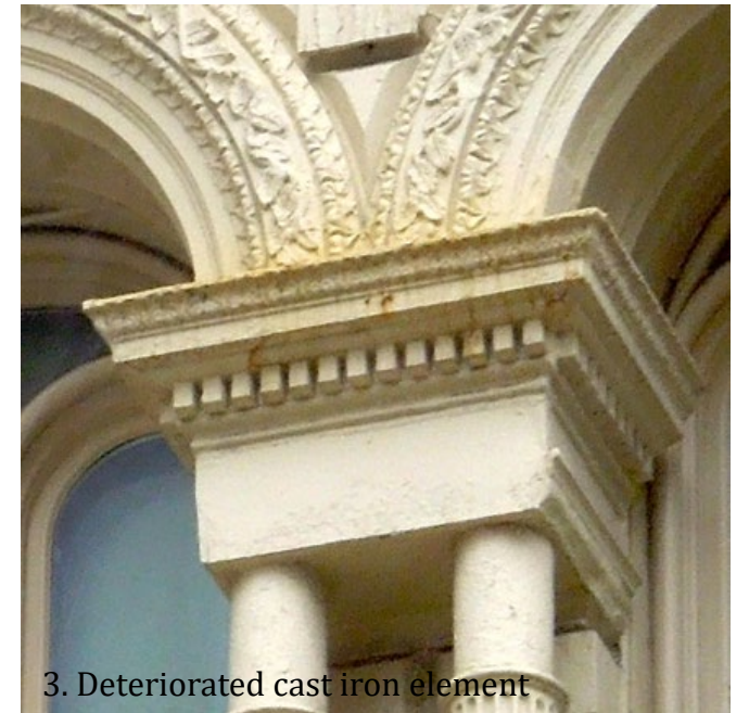
4. Rusted cast iron element.
