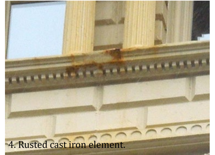
5. Damaged cast iron element.
