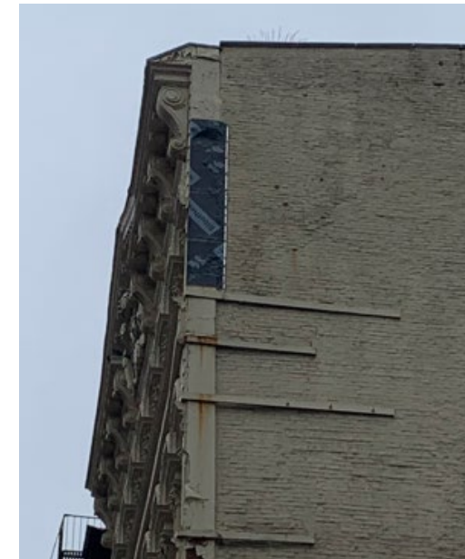
Church St - Southeast corner missing cast iron element . Replacement to match Northeast corner design.
