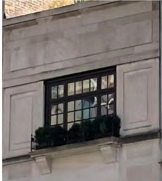
2. TOP WOOD WINDOW (NOT HISTORIC)
