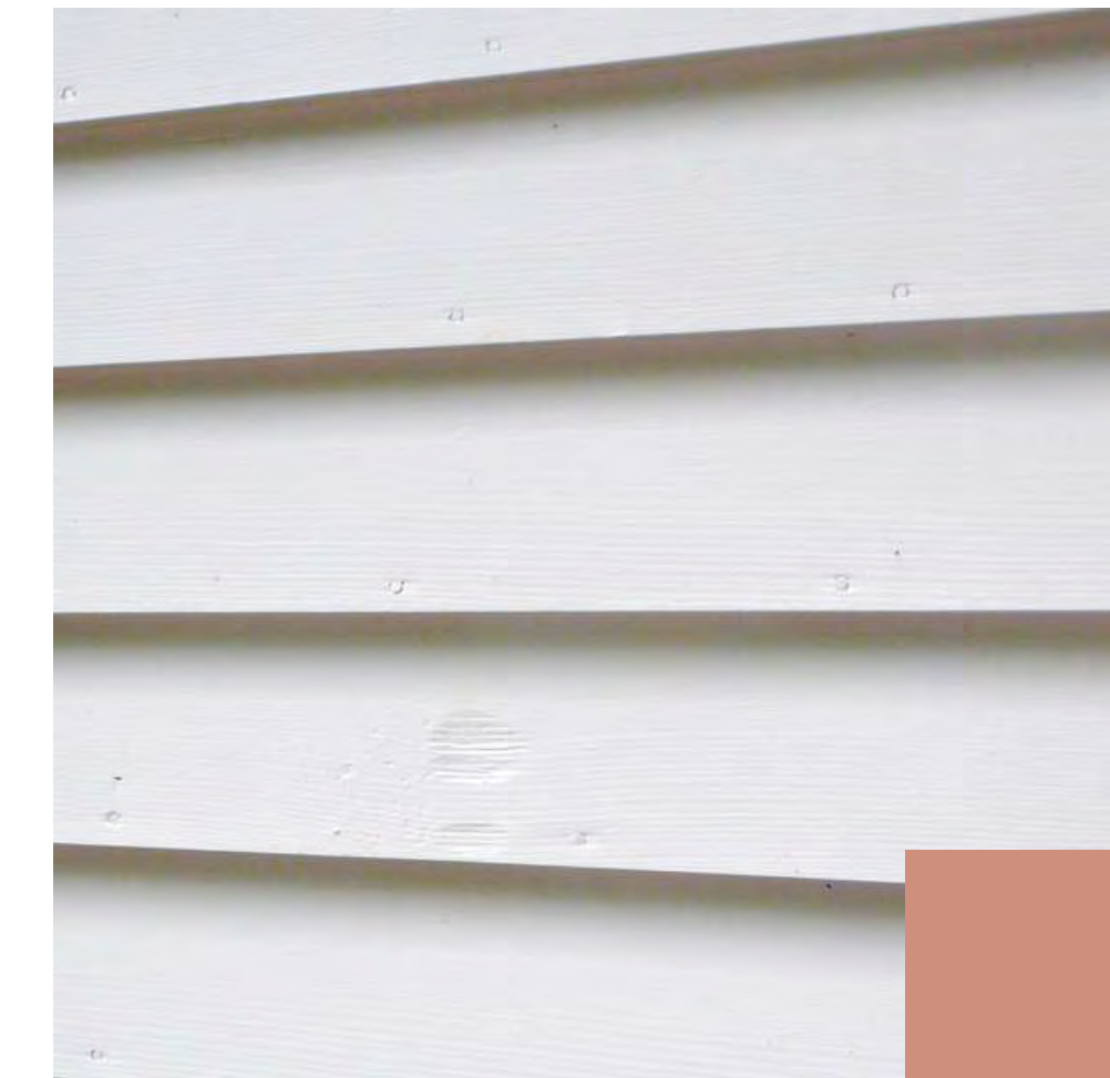
NEW REAR FACADE DORMER CALP BOARD DESIGN TO MATCH EXISTING DORMER AT FRONT FACADE. COLOR TO MATCH EXISTING FRONT FACADE DORMER
