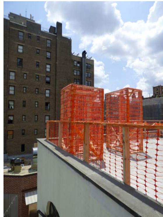
5 | Mechanical units and railing, looking east
