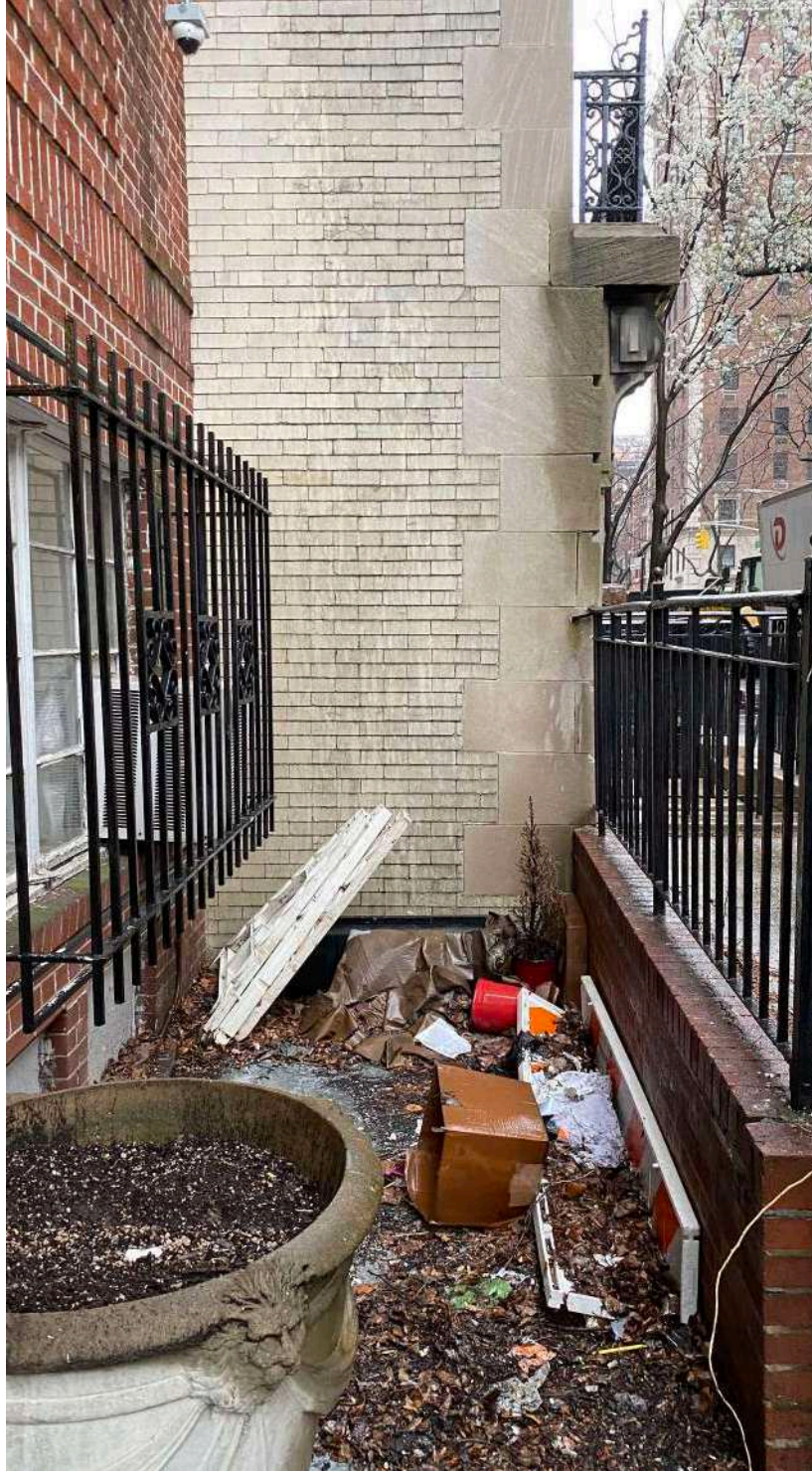
TRASH AND DEBRIS GATHERING AT CURRENT ENTRY
