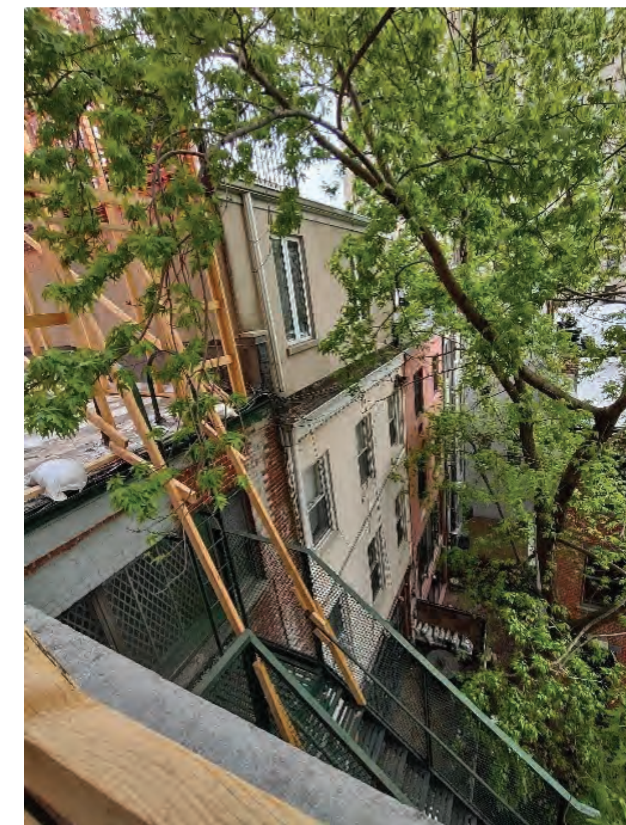
PHOTO 3: 1211 PARK AVENUE CARNEGIE HILL HISTORIC DISTRICT ROOFTOP ADDITION. ADDITION IS IN THE SAME PLANE AS REAR FACADE
