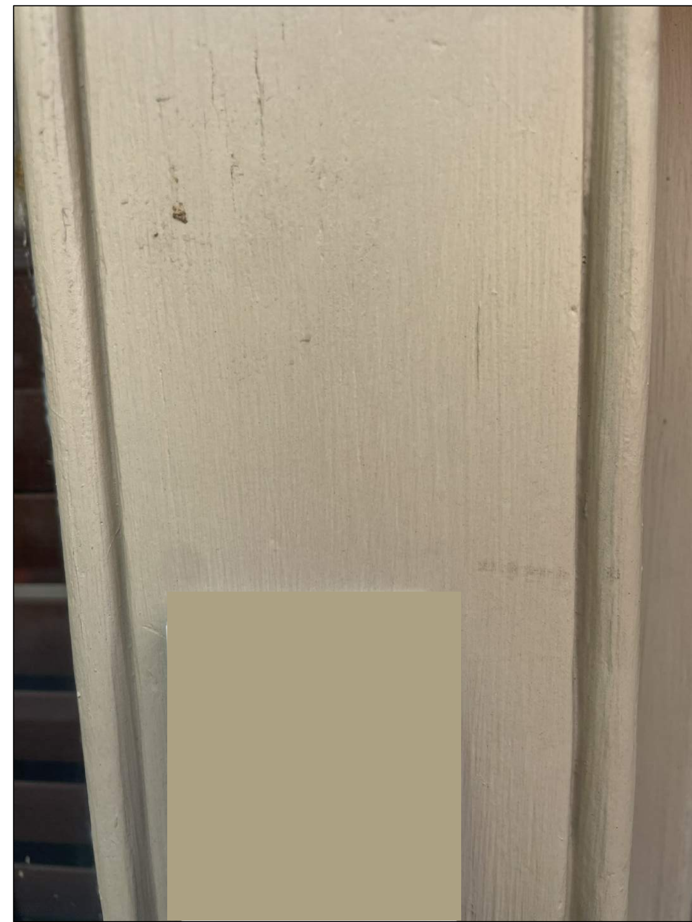
2 EXISTING WINDOW COLOR & MARVIN CUSTOM COLOR BASED ON BENJAMIN MOORE HC98 NTS
