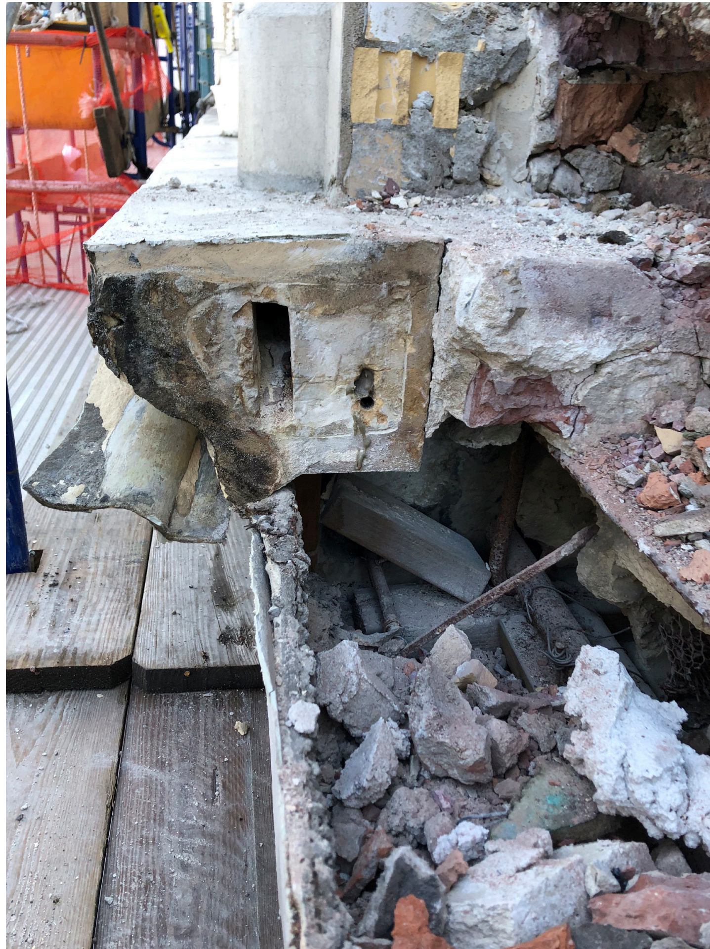
Cross-Section View of Balcony showing detached metal tie rods and cracked terracotta
