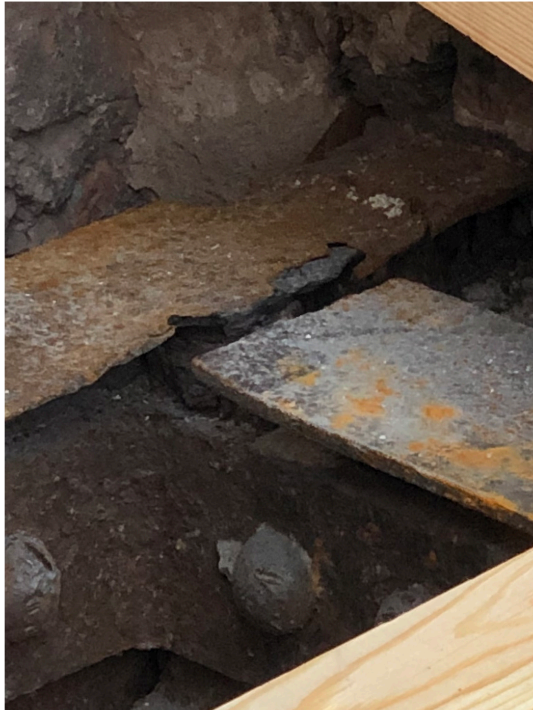
Existing Balcony Structural Deterioration: Outrigger Completely Detached From C-Channel
