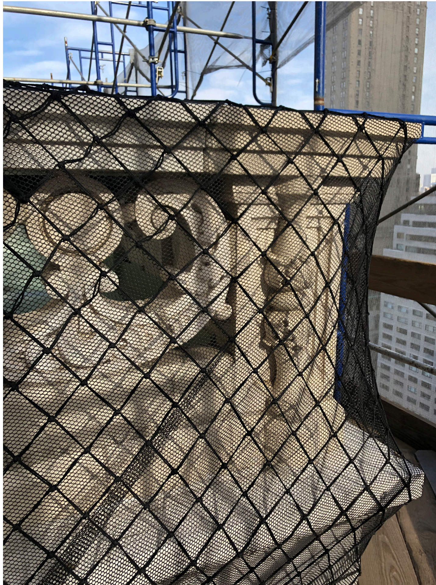
Current Balcony Condition at Grand Army Plaza- Protective Netting Around Deteriorated Terracotta
