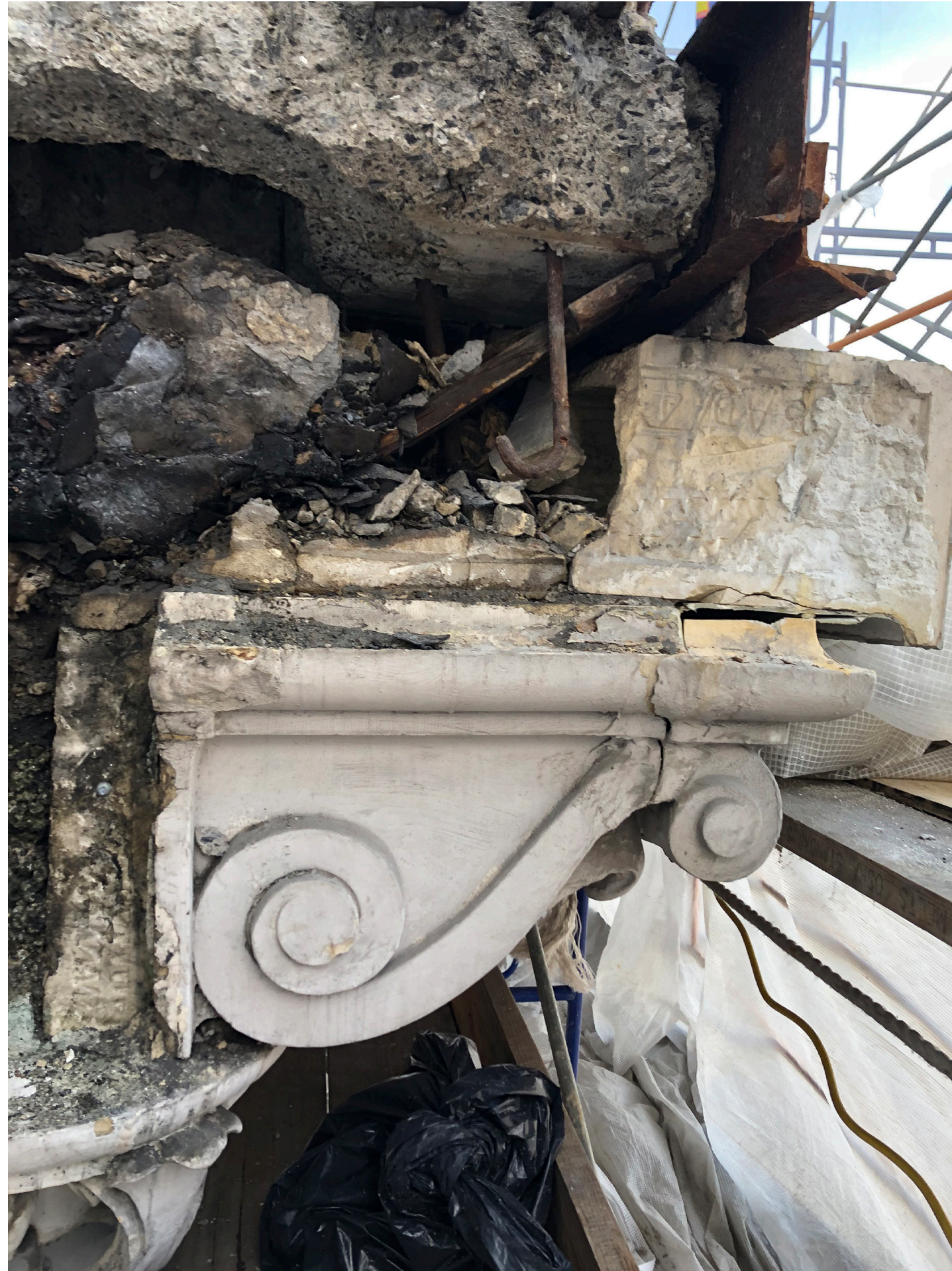
Cross-Section View of Balcony showing detached metal tie rods and cracked terracotta
