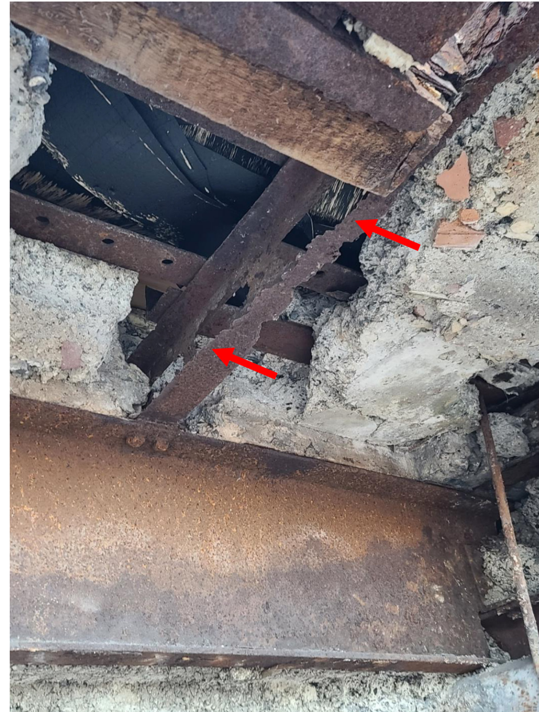
Typical Condition of Outrigger Beam Supporting the Balcony Deck and Terracotta Super Structure. Section was Formerly a W8" x3" Beam
