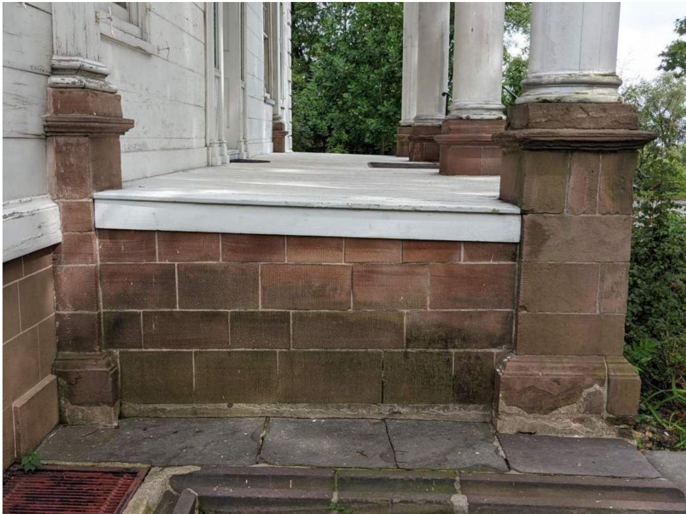
16. View of West side of South porch. Note: Pitch of the existing porch exceed the maximum slope for an ADA accessible approach.
