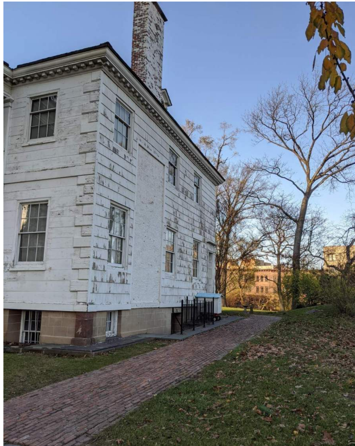
8. View of approach to East Entrance from South side of mansion and bluestone plaza. Note adjacent grade change and rock outcropping
