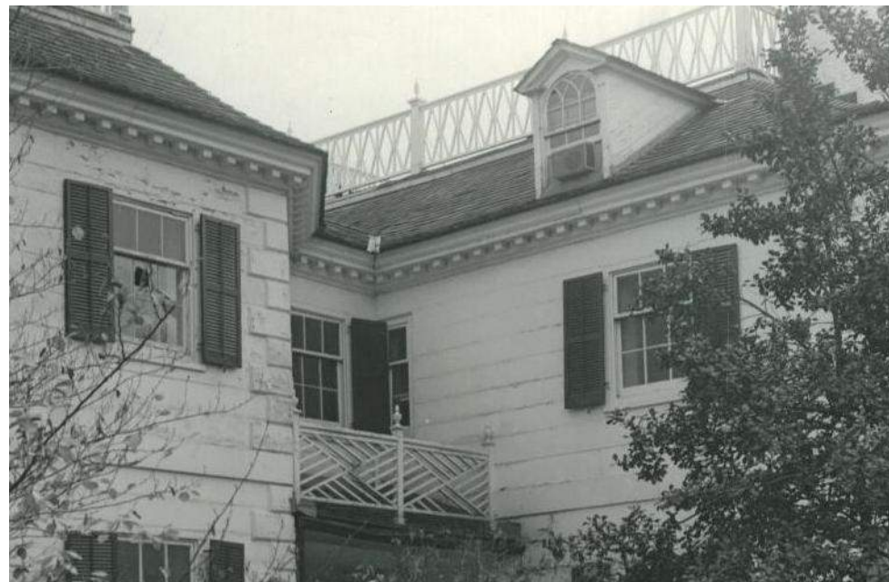
Aerial view of missing roof railings, C. 1934, Olmsted Archives
