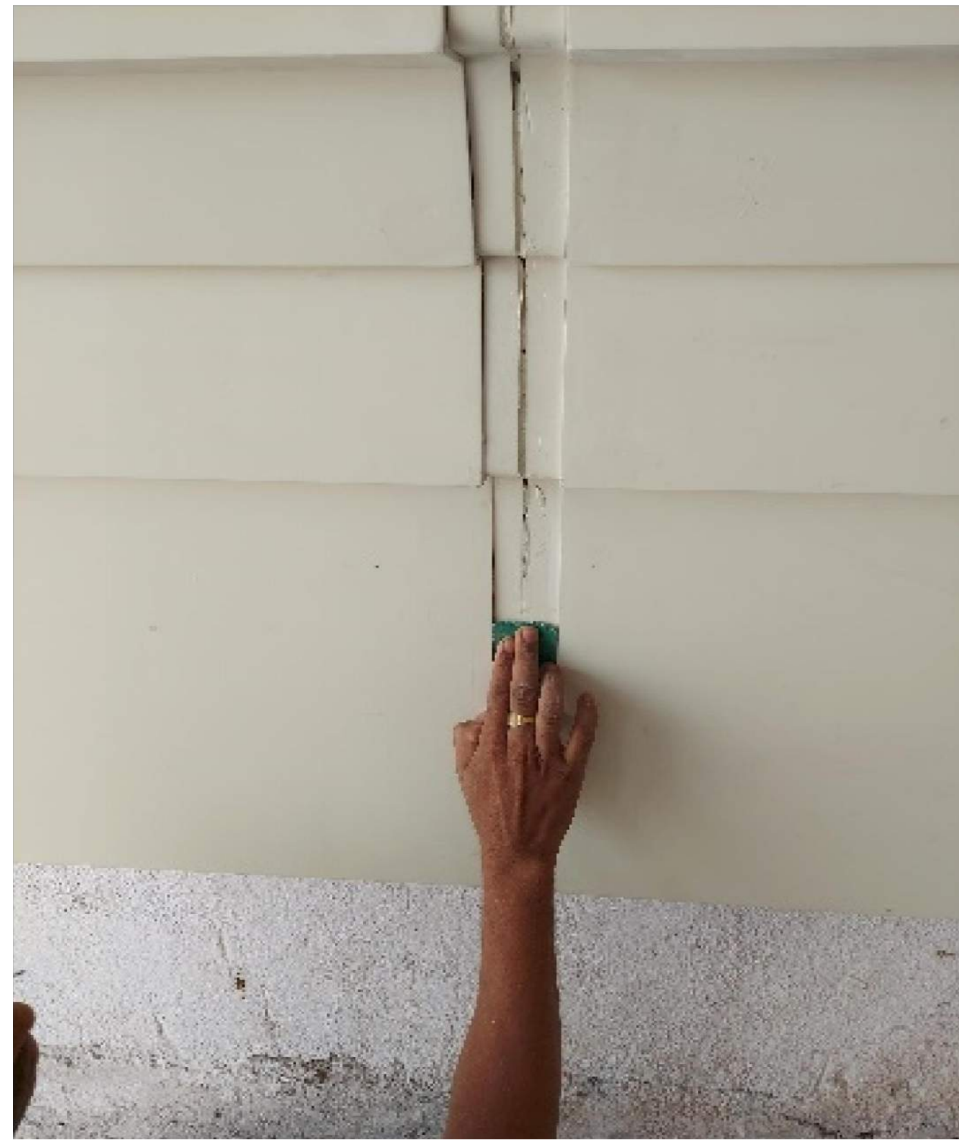
1. SAND AREA BETWEEN PANELS
