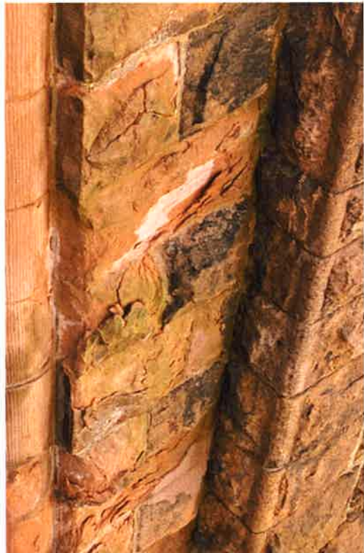
North Tower – Spalled Stones
