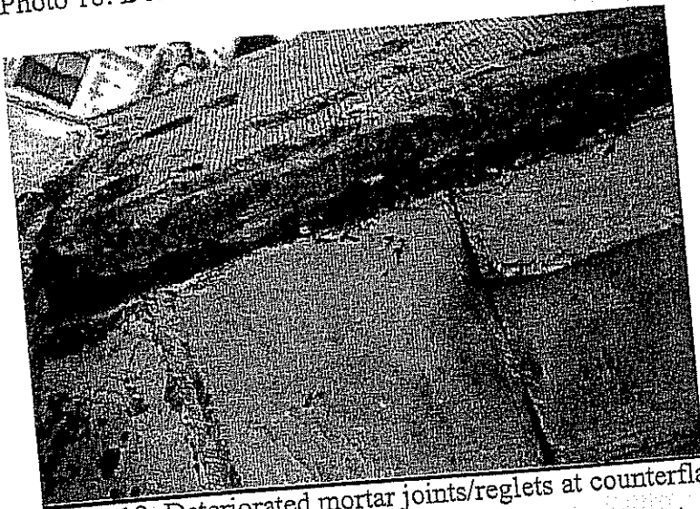
Photo 18: Deteriorated mortar joints/reglets at counterflashing.
