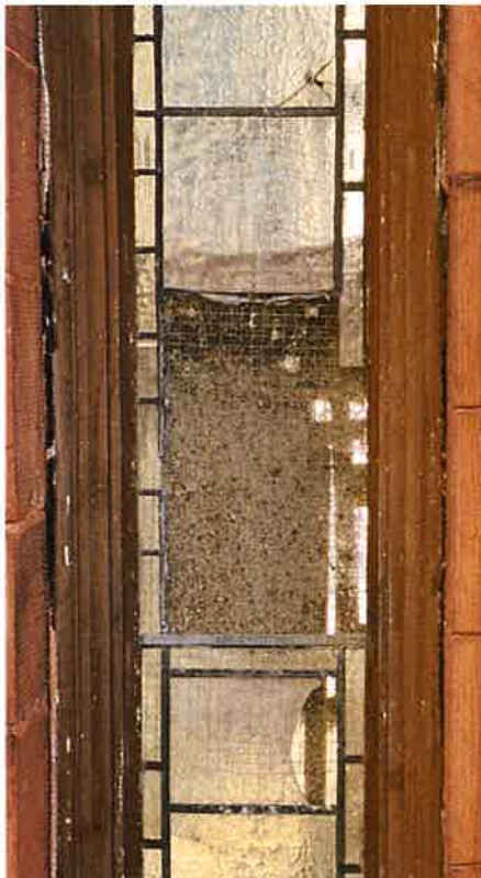
North Tower – Window Deteriorated
