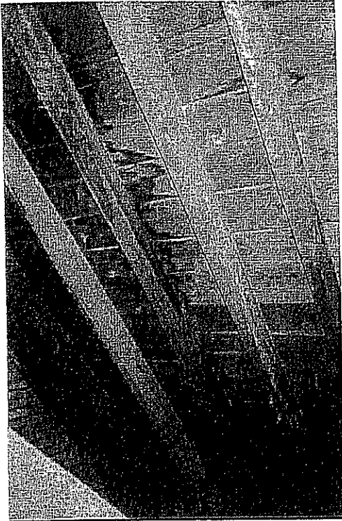
Photo 1: Water staining at roof planks, typical.
