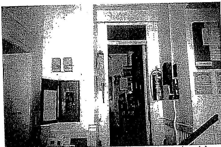
Photo M16: View of additional ducts and fan serving the sides of church and crawl space.
