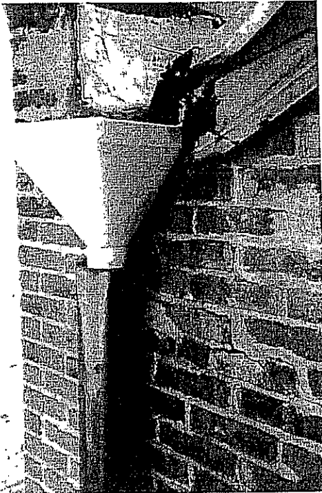
Photo 40: Leader and downspout no longer connected at northeast corner.
