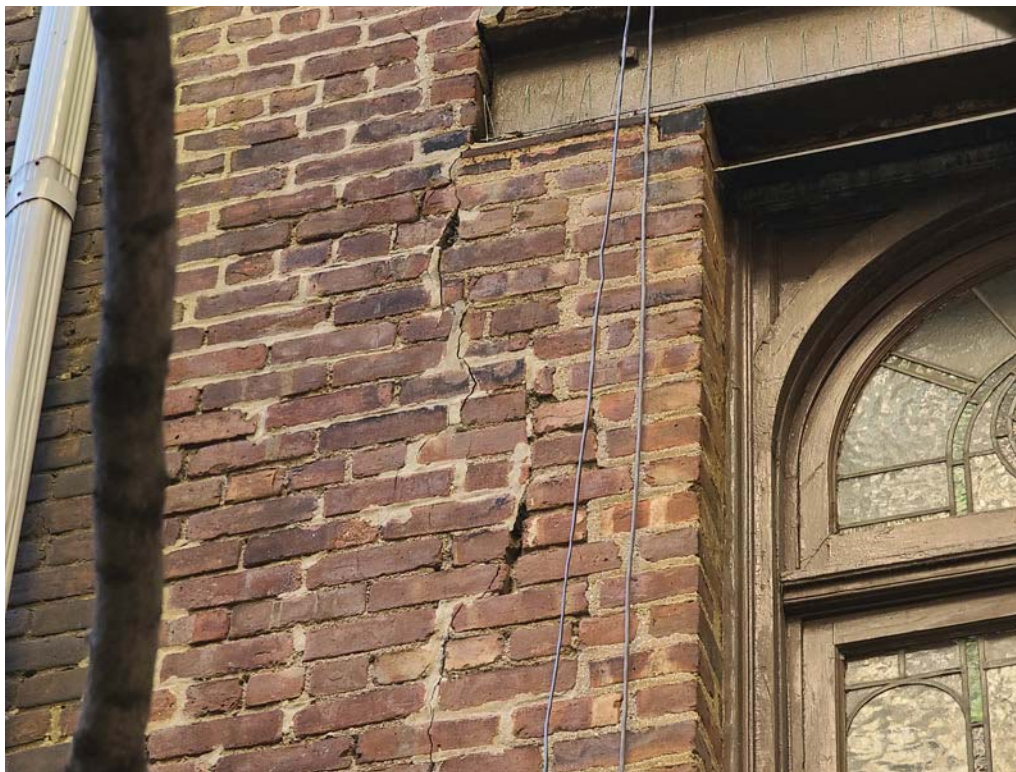
PHOTO 4: CRACKS IN BRICK EXTERIOR BEARING WALL
