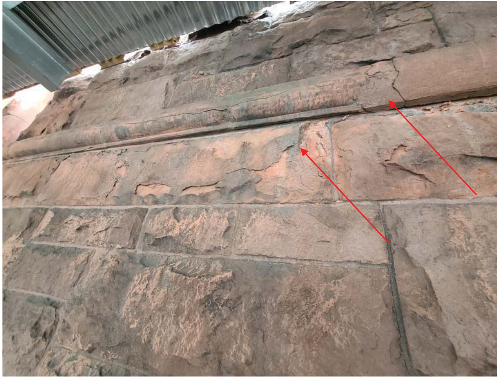
PHOTO 3: TYPICAL FACADE CONDITION
