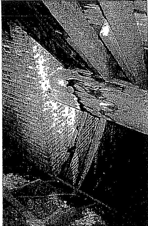
Photo 8: Water stains run down masonry walls at southeast stair tower.
