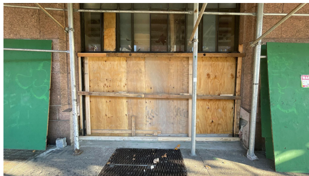
EXISTING MISSING DOOR
