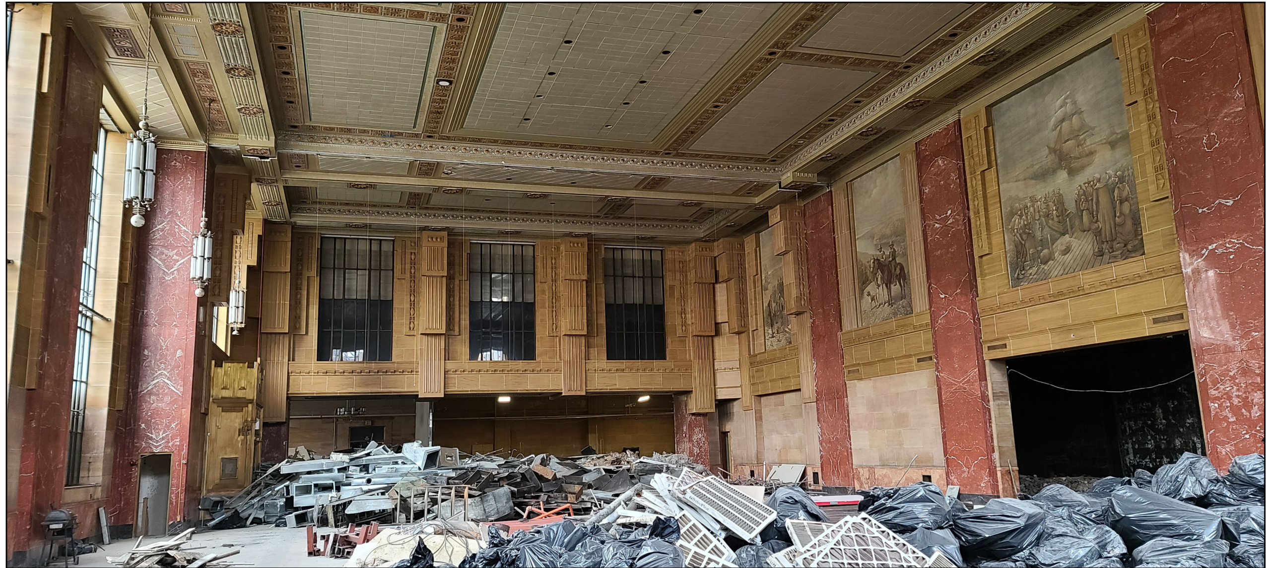
DEBRIS REMOVAL FROM BASEMENT FLOOD DAMAGE
