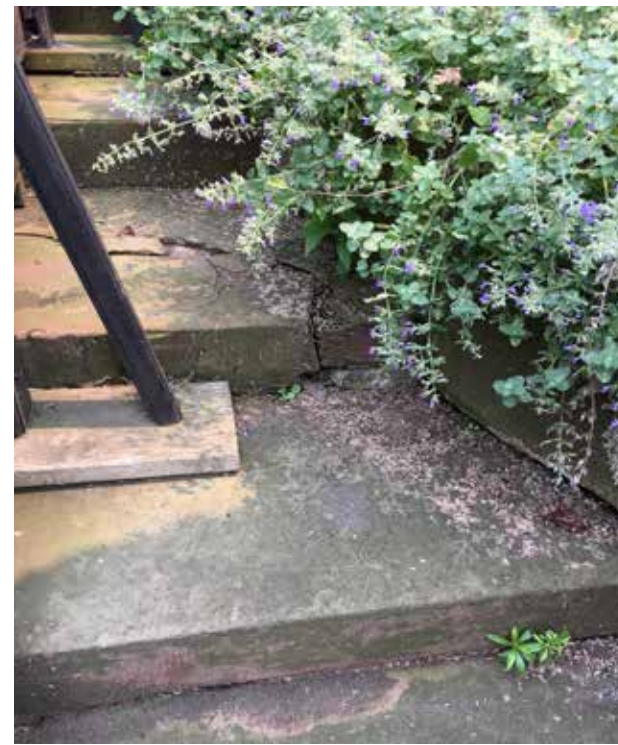
Typical isolated spalling at the brownstone steps.
