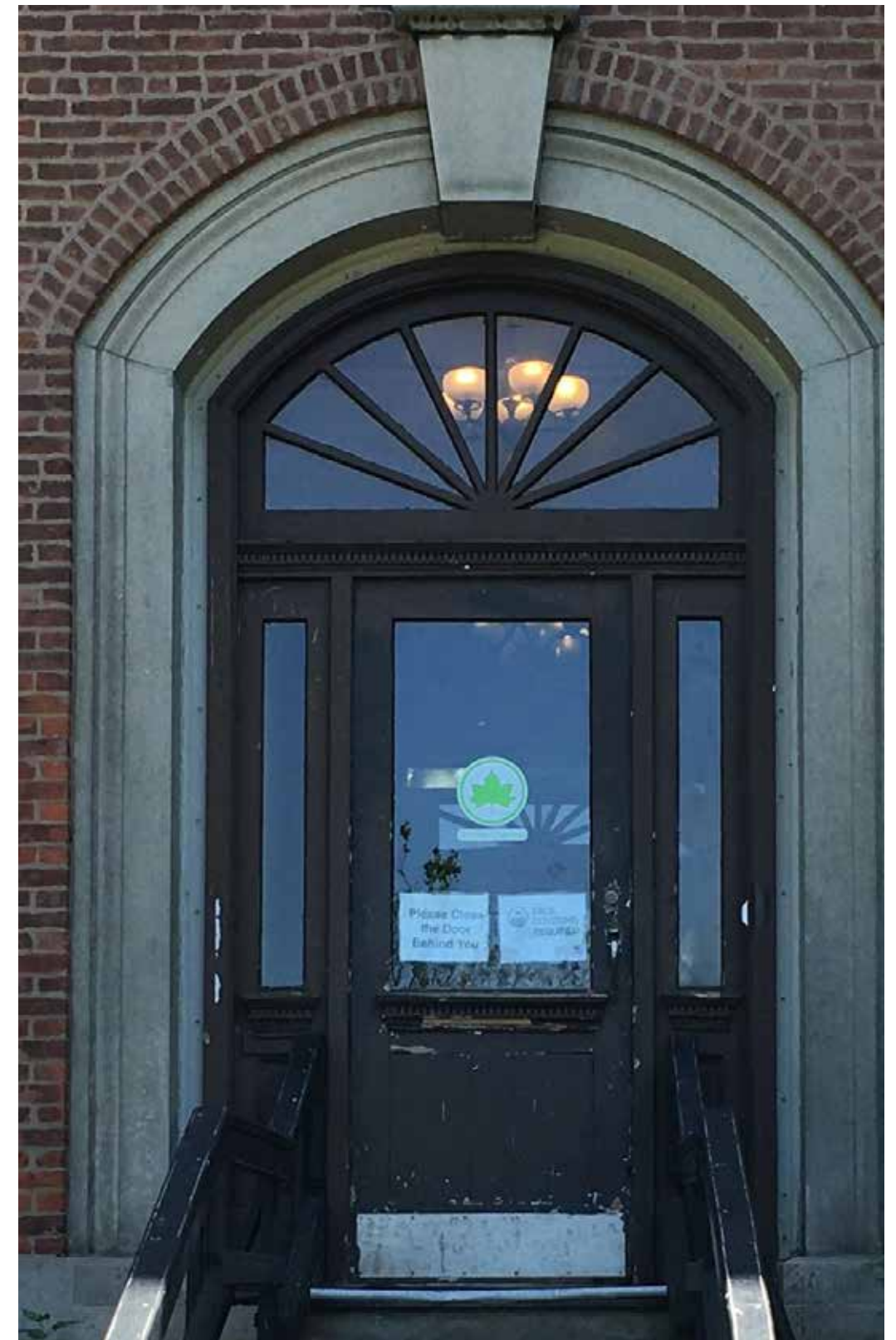
Based on historic photographs, the existing door was installed in the 1930s.
