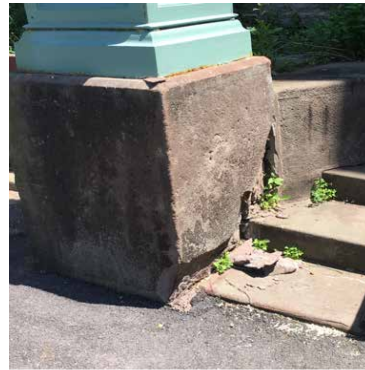
Spalling and scaling at the brownstone piers.
