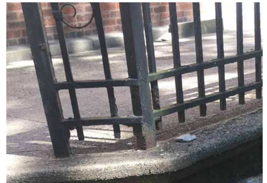
Painted black steel fence is not properly maintained; corroded and chipping.
