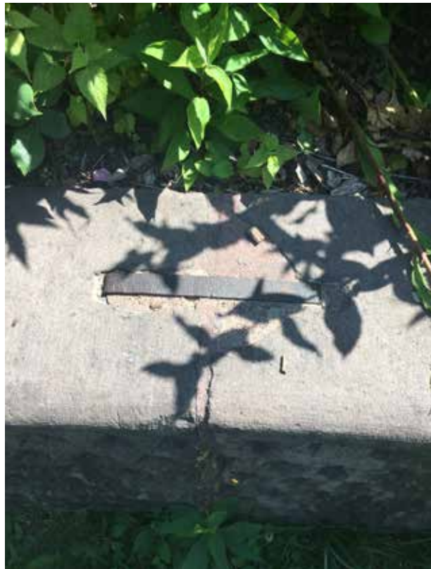
Iron staples on brownstone wall, not original.
