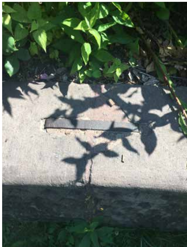
Iron staples on brownstone wall, not original.
